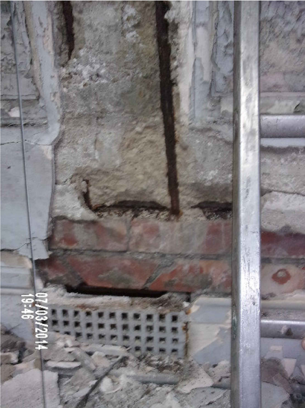
DAMAGED CONCRETE PHOTO (NTS)
