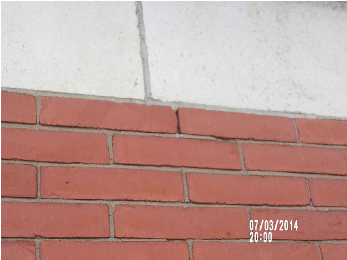
REPOINTING OF BRICKWORK REQUIRED (NTS)
