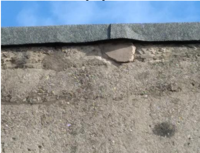
Example of lifted felt at edge of roof of garages. Close inspection found these areas to be shallow and heavily cobwebbed indicating a lack of recent bat activity
