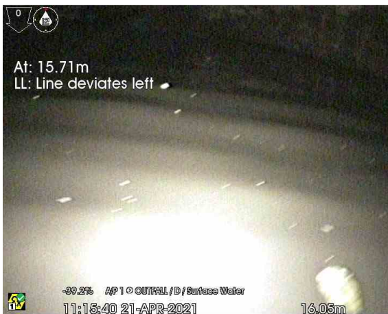
1_16-05m_111540.jpg, 00:02:06, 16.05 m Line deviates left
