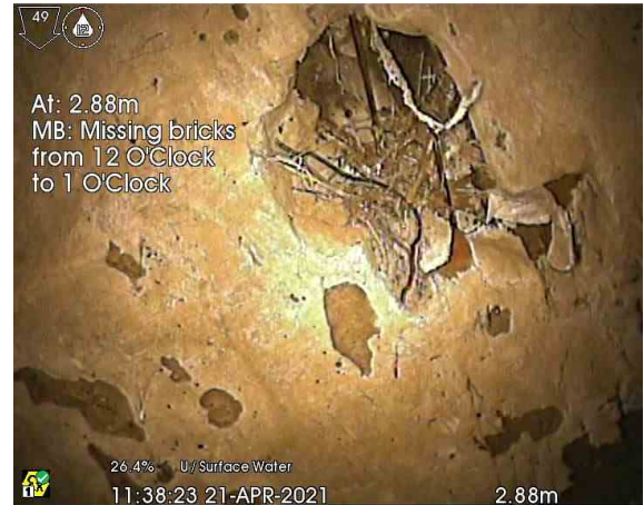
2_2-88m_113823.jpg, 00:00:40, 2.88 m Missing bricks from 12 o'clock to 1 o'clock
