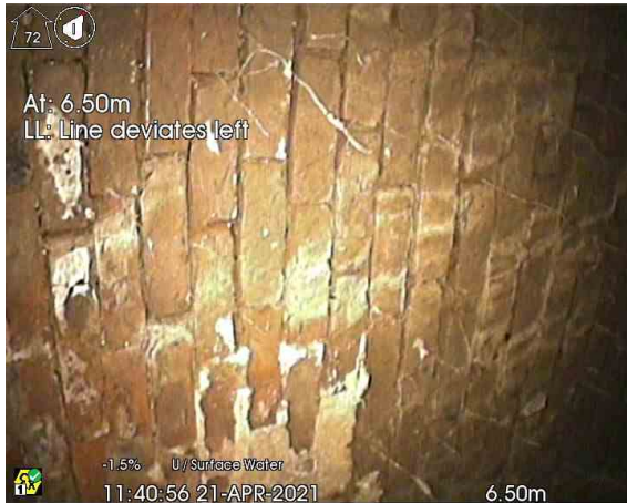
2_6-50m_114056.jpg, 00:02:26, 6.50 m Line deviates left
