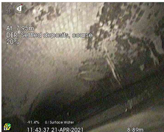
2_8-89m_114337.jpg, 00:04:42, 8.89 m Settled deposits, coarse, 20% cross-sectional area loss
