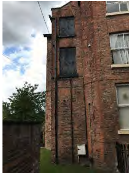
Boarded up windows
