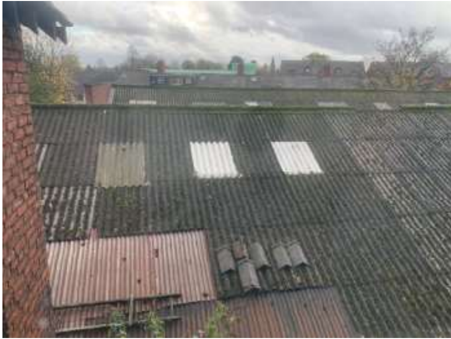
Figure 08: Existing Garage Asbestos Roofing (Phase 1 Desk Study)
