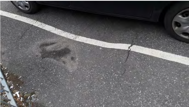
Photograph 4 (P4) Evidence of localised subsidence and cracking of tarmacadam in the car park.
