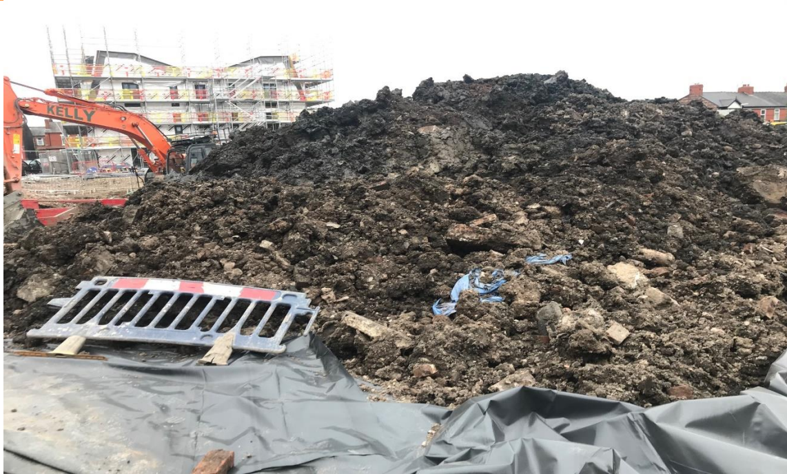
PLATE 29 – IMPACTED MATERIAL BENEATH SUBSTATION
