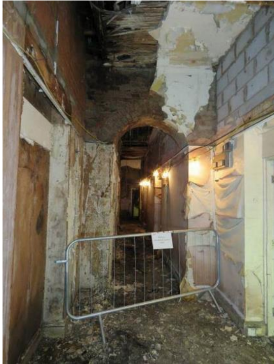
Figure 113: Looking south along the first floor central corridor, showing the 1977 alterations and water damage (Room F13). (Source: SLHA 2017)
