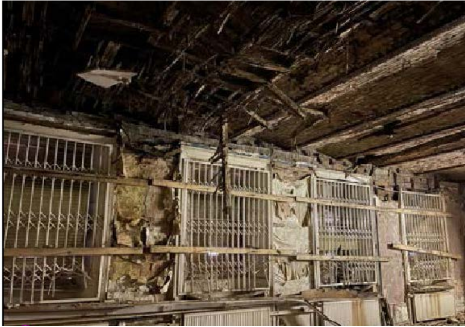
Figure 106: Room G23 (looking south-east) as seen in 2022 – This large room shows the complete loss of original lath and plaster ceiling, with only a small fragment of cornice left to the south-west corner due to substantial damage caused by water ingress (Source: Snook Architects 2022).
