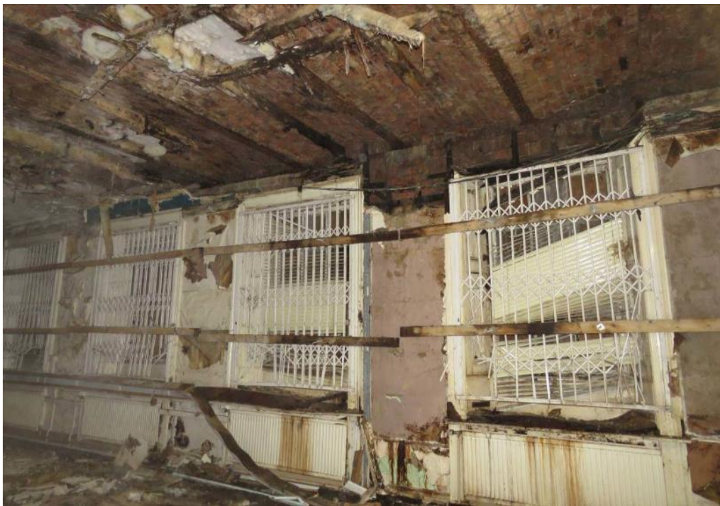
Figure 105: Room G23 (looking east) – This view shows the original jack-arch construction of the ground floor ceiling, which was originally covered with a suspended lath and plaster ceiling with deep cornice (now mostly collapsed due to water ingress. Note the original shutters to window reveals, intended to provide additional security to the canal company's documents (Source: SLHA 2017)
