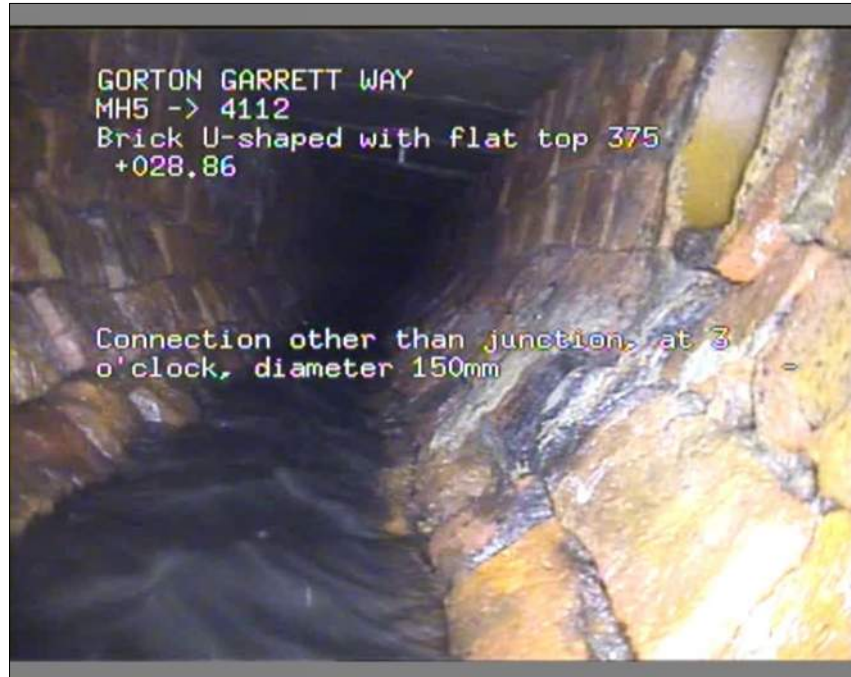
Photo: 4_4_27_A.JPG 28.84m, Connection other than junction, at 3 o'clock, diameter 150mm
