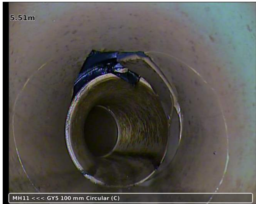
Photo: 20181123-144743-snap0003.jpg 5.51m, Broken pipe at joint from/at 10 o'clock to 02 o'clock
