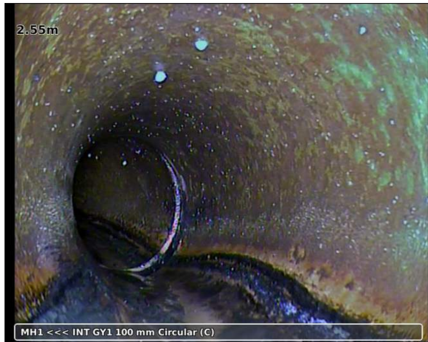
Photo: 20181122-102339-snap0003.jpg 2.55m, Line deviates left
