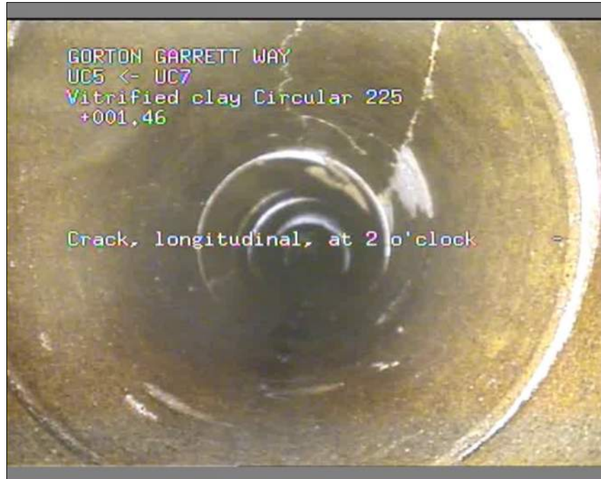
Photo: 15_15_85_A.JPG 1.46m, Crack, longitudinal, at 2 o'clock
