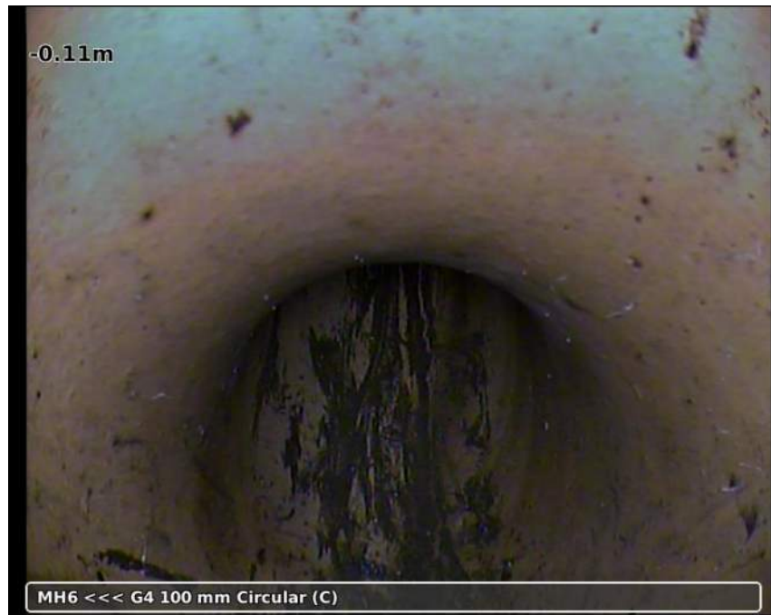
Photo: 20181123-082900-snap0001.jpg -0.11m, Line deviates up
