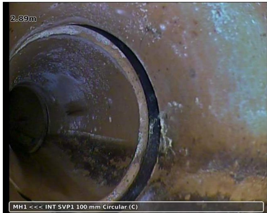
Photo: 20181122-102650-snap0003.jpg 2.89m, Line deviates left
