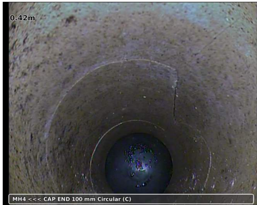
Photo: 20181122-120552-snap0003.jpg 0.42m, Crack circumferential from/at 12 o'clock to 12 o'clock
