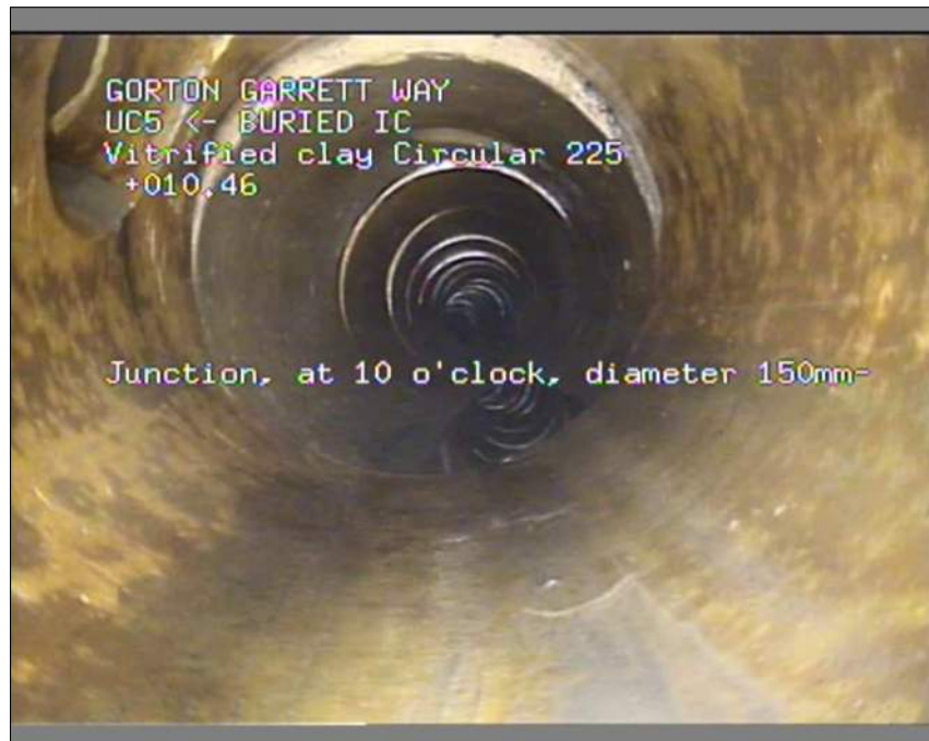
Photo: 13_13_80_A.JPG 10.42m, Junction, at 10 o'clock, diameter 150mm
