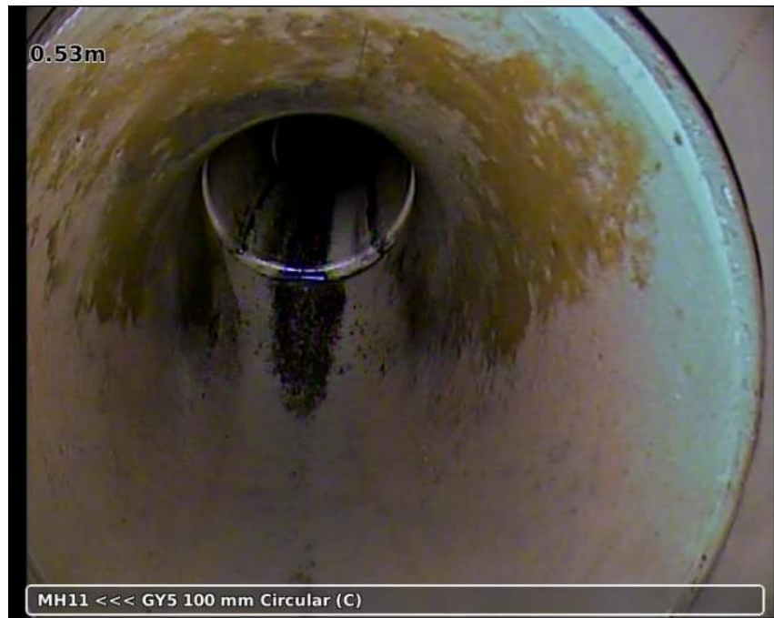
Photo: 20181123-144743-snap0001.jpg 0.53m, Line deviates up
