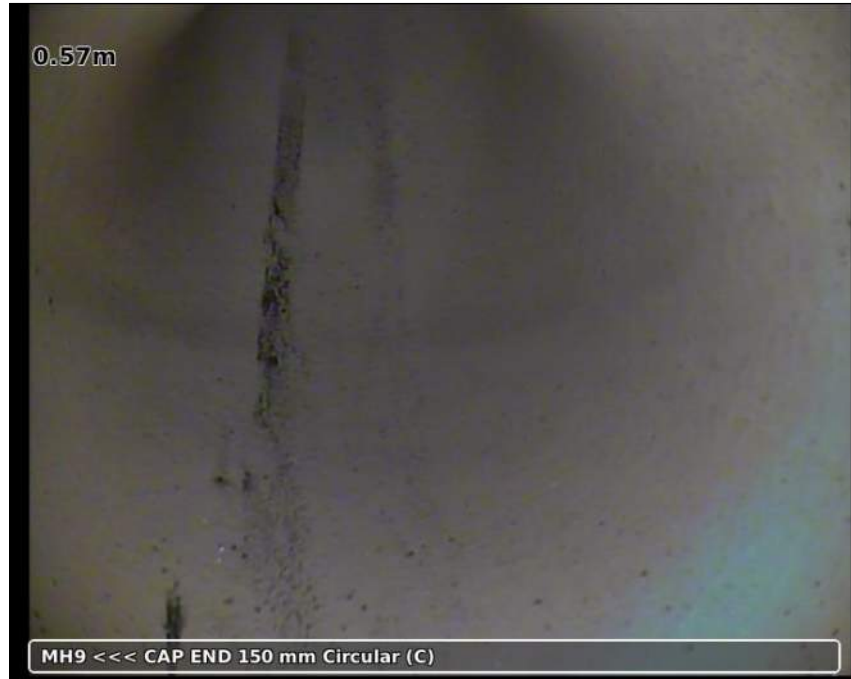
Photo: 20181123-115736-snap0002.jpg 0.57m, Line deviates up
