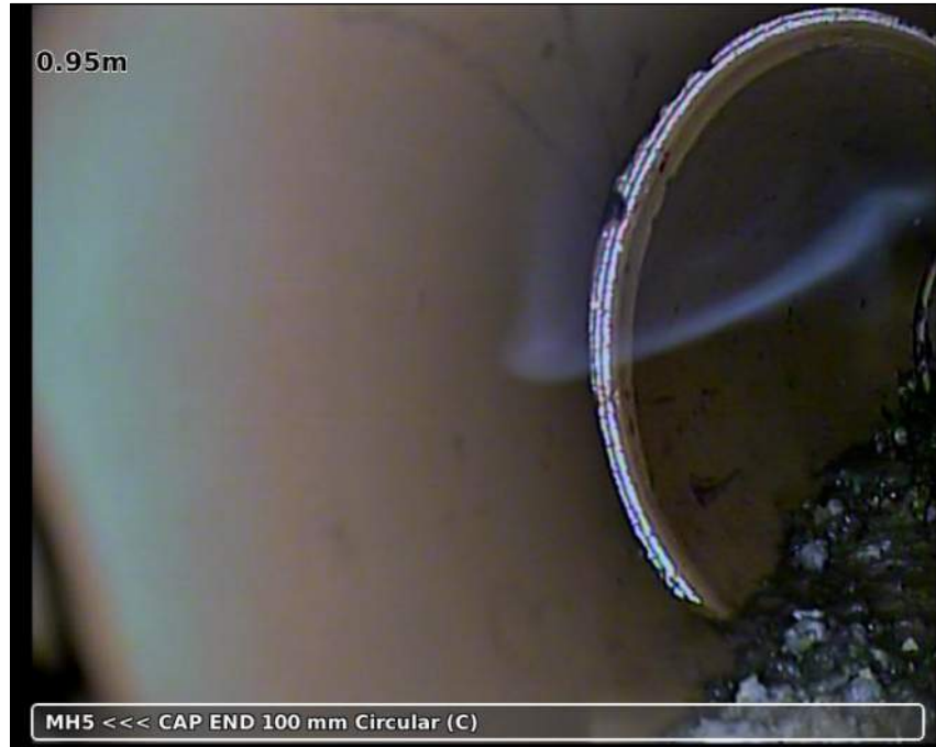
Photo: 20181123-100650-snap0002.jpg 0.95m, Attached deposits encrustation from/at 05 o'clock to 07 o'clock 10 % cross-sectional area loss
