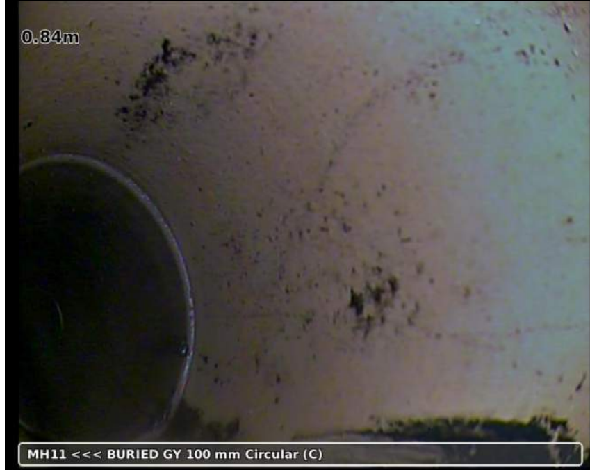
Photo: 20181123-141150-snap0002.jpg 0.84m, Line deviates left
