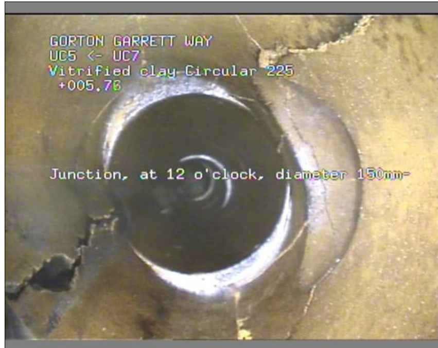
Photo: 15_15_90_A.JPG 5.76m, Junction, at 12 o'clock, diameter 150mm
