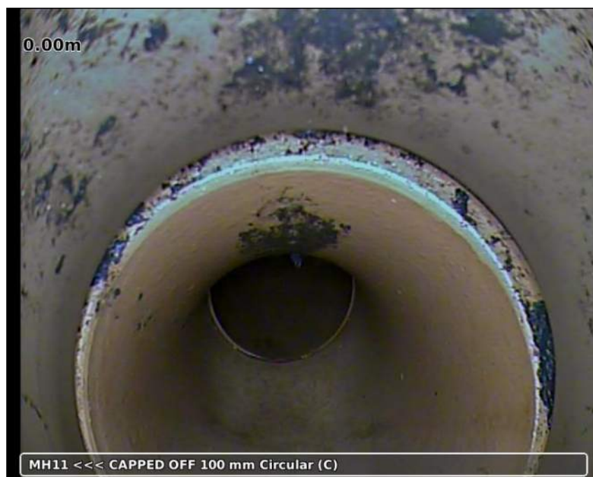
Photo: 20181123-135029-snap0001.jpg 0m, Line deviates up
