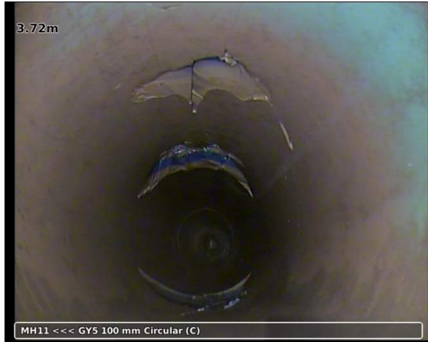
Photo: 20181123-144743-snap0002.jpg 3.72m, Hole in drain or sewer from/at 11 o'clock to 01 o'clock
