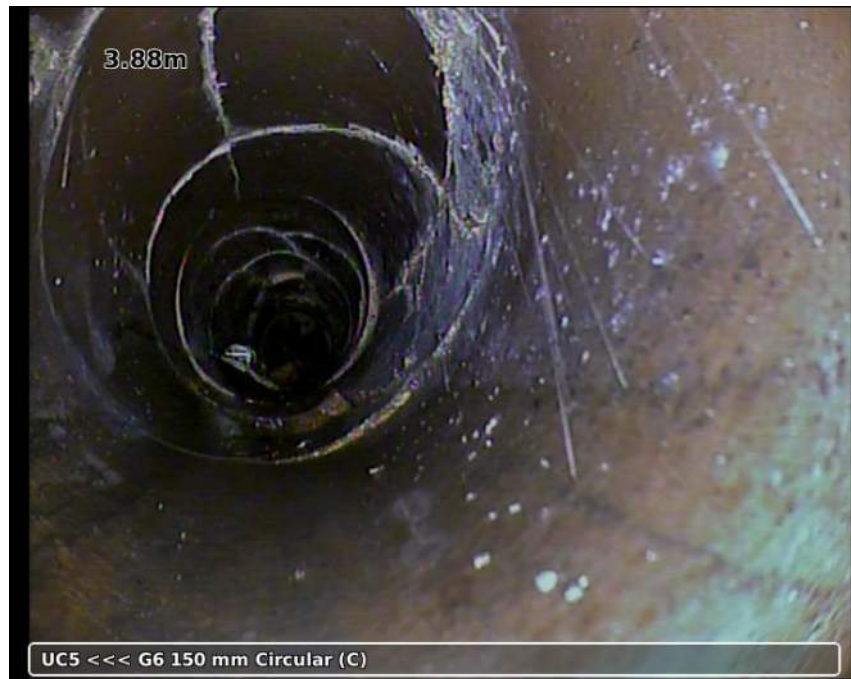
Photo: 20181204-144214-snap0003.jpg 3.88m, Fracture multiple from/at 12 o'clock to 12 o'clock
