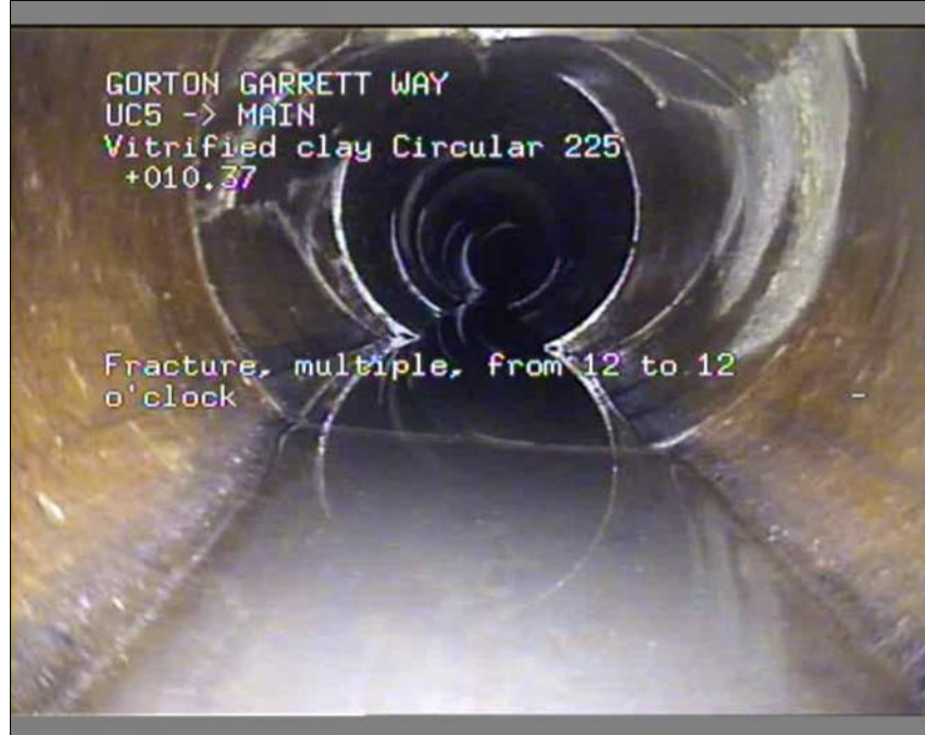
Photo: 12_12_69_A.JPG 10.37m, Fracture, multiple, from 12 to 12 o'clock
