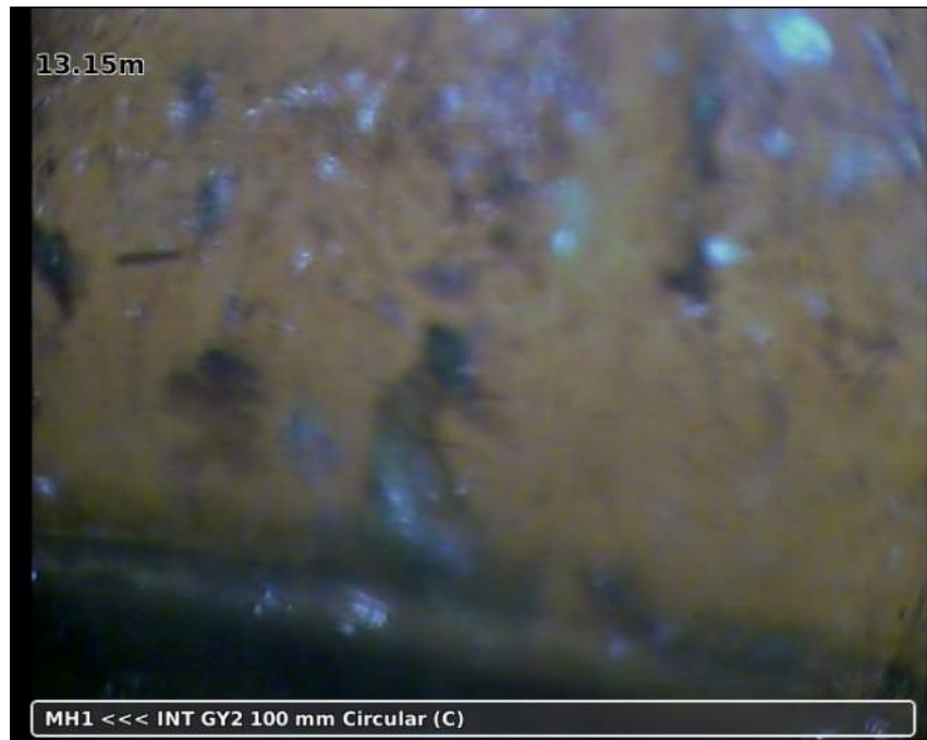
Photo: 20181122-103009-snap0005.jpg 13.15m, Finish node type gully reference number: INT GY2
