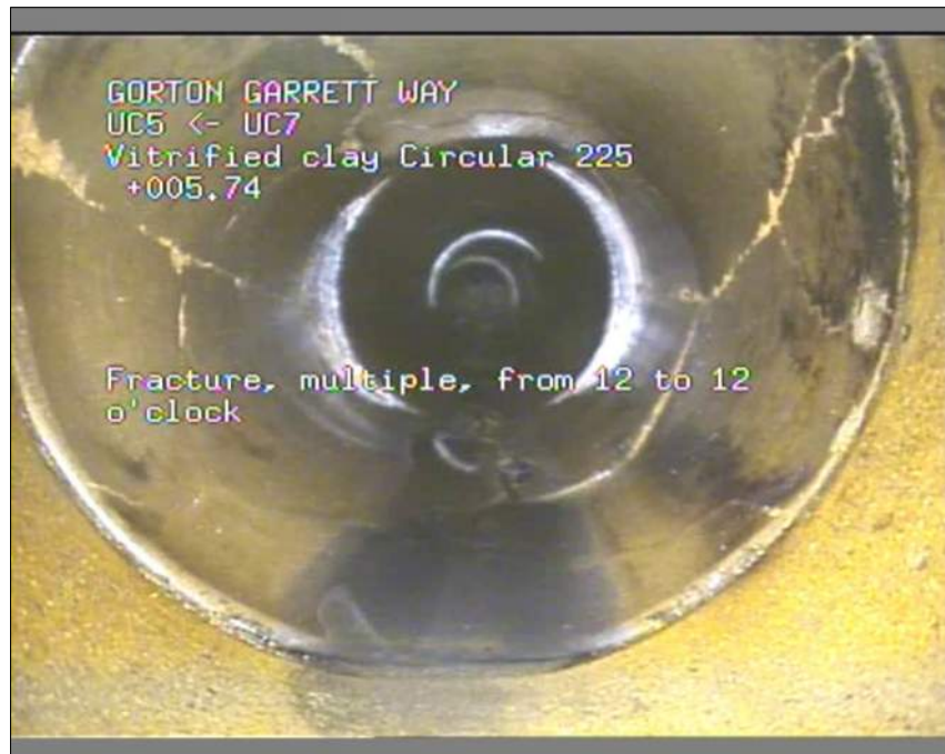
Photo: 15_15_89_A.JPG 5.74m, Fracture, multiple, from 12 to 12 o'clock
