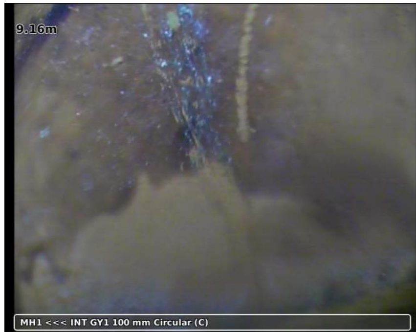
Photo: 20181122-102339-snap0005.jpg 9.16m, Finish node type gully reference number: INT GY1
