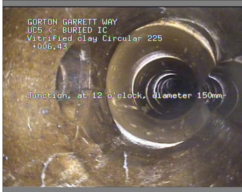
Photo: 13_13_79_A.JPG 6.43m, Junction, at 12 o'clock, diameter 150mm
