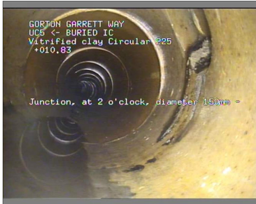
Photo: 13_13_81_A.JPG 10.83m, Junction, at 2 o'clock, diameter 150mm
