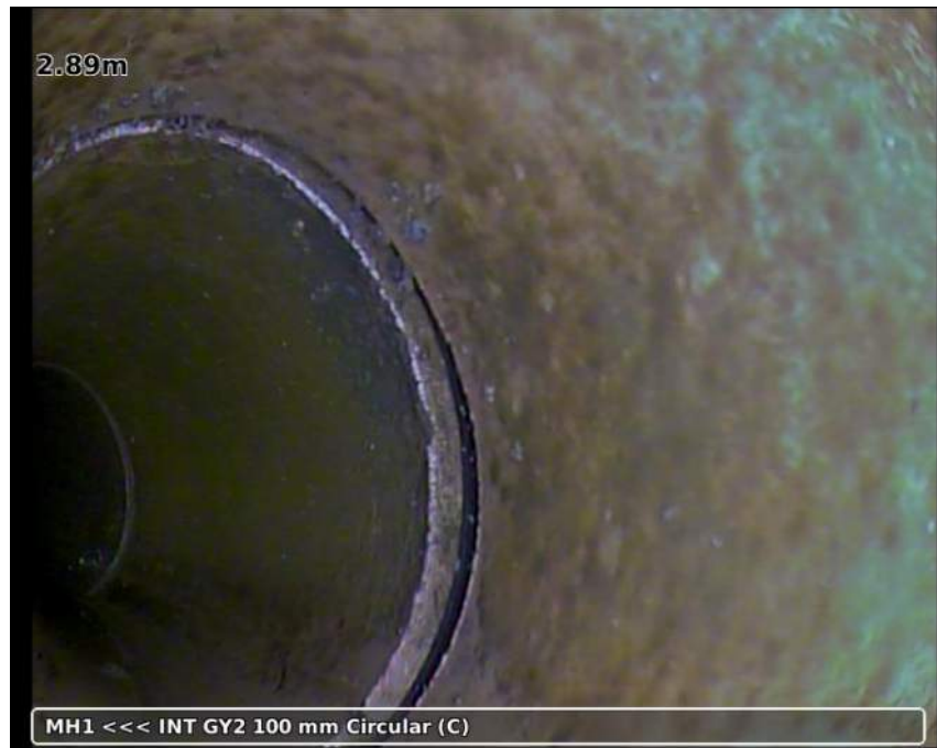
Photo: 20181122-103009-snap0003.jpg 2.89m, Line deviates left
