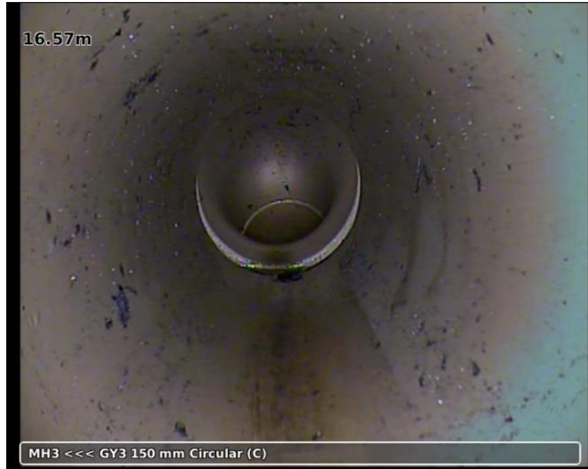
Photo: 20181122-114351-snap0002.jpg 16.57m, Line deviates up
