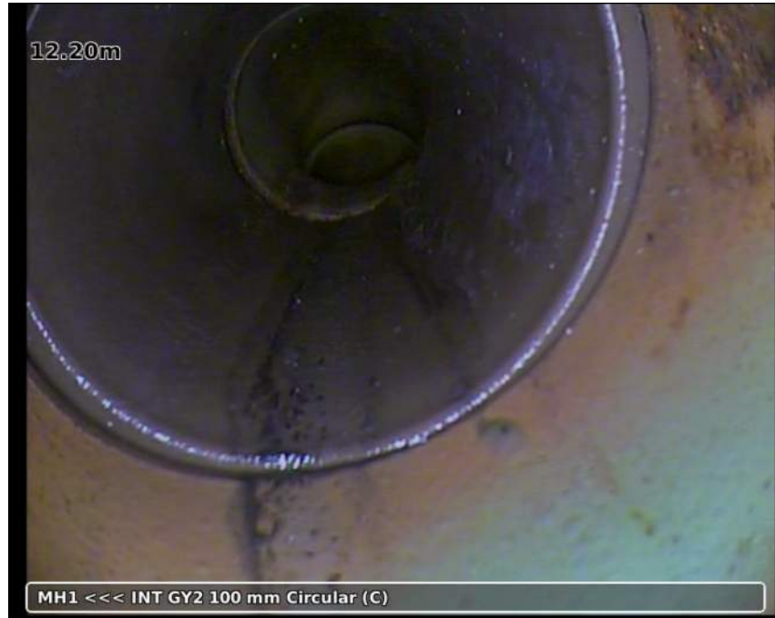
Photo: 20181122-103009-snap0004.jpg 12.2m, Line deviates up
