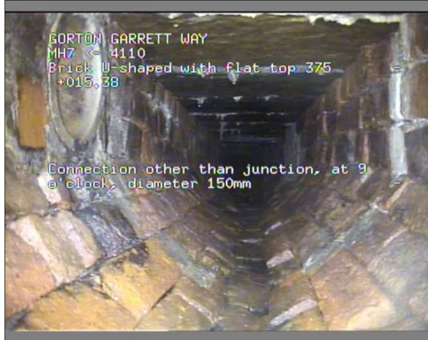
Photo: 3_3_18_A.JPG 15.38m, Connection other than junction, at 9 o'clock, diameter 150mm
