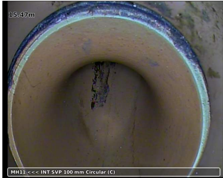
Photo: 20181123-142115-snap0004.jpg 15.47m, Line deviates up
