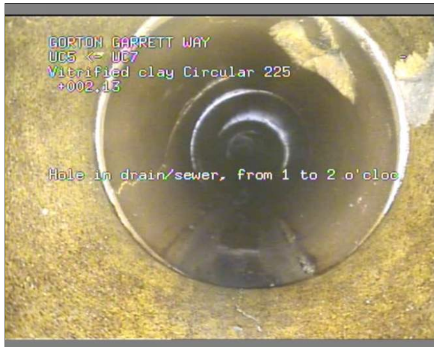
Photo: 15_15_86_A.JPG 2.13m, Hole in drain/ sewer, from 1 to 2 o'clock
