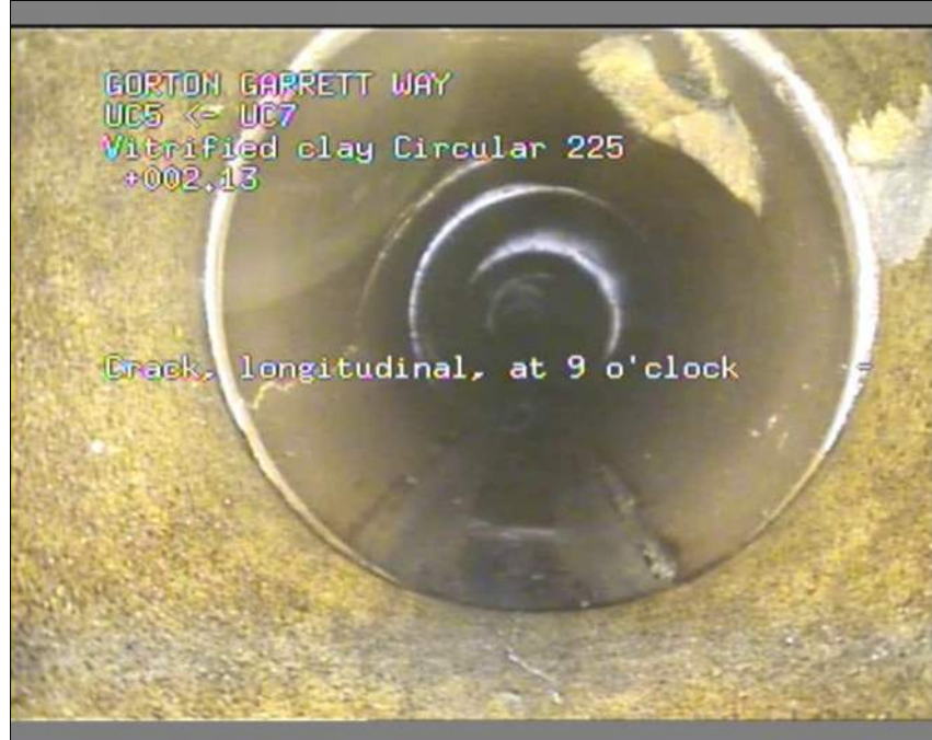
Photo: 15_15_88_A.JPG 2.13m, Crack, longitudinal, at 9 o'clock
