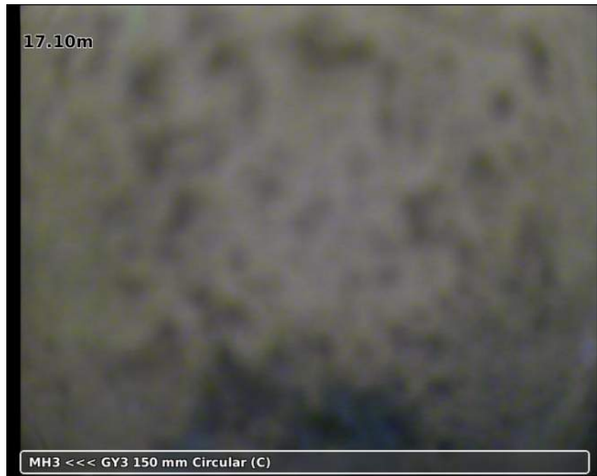
Photo: 20181122-114351-snap0003.jpg 17.1m, Finish node type gully reference number: GY3
