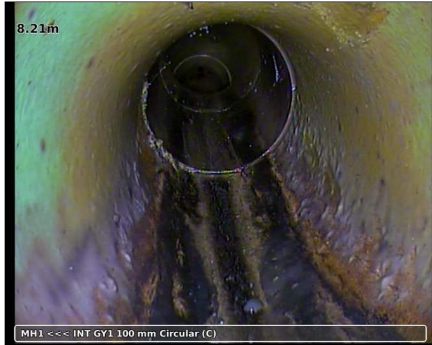
Photo: 20181122-102339-snap0004.jpg 8.21m, Line deviates up
