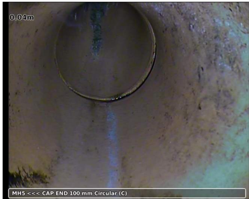
Photo: 20181123-100650-snap0001.jpg 0.04m, Line deviates up
