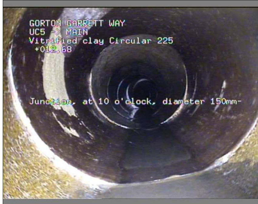
Photo: 12_12_71_A.JPG 12.68m, Junction, at 10 o'clock, diameter 150mm
