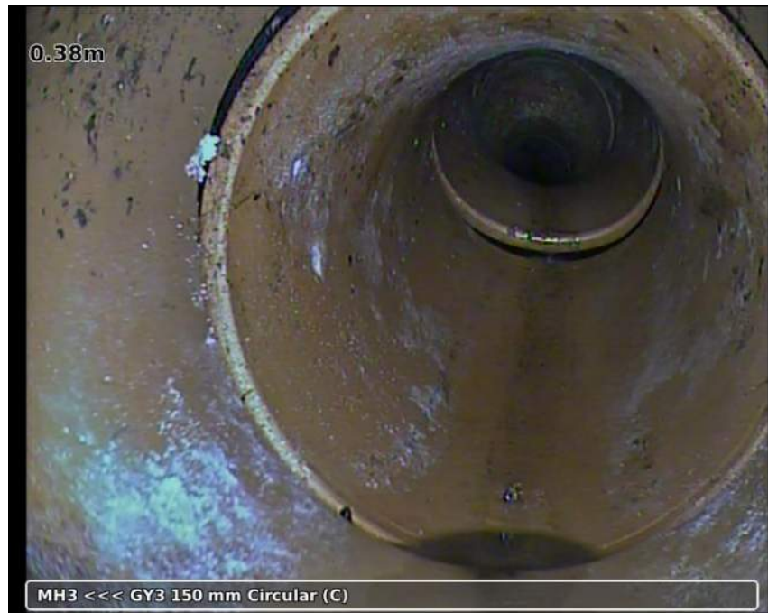
Photo: 20181122-114351-snap0001.jpg 0.38m, Line deviates up
