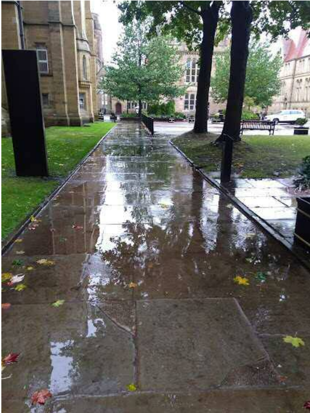
Fig 1: Taken from Beyer entrance - ponding on the path to the Beyer Building & temporary cement repairs to the stone flags
