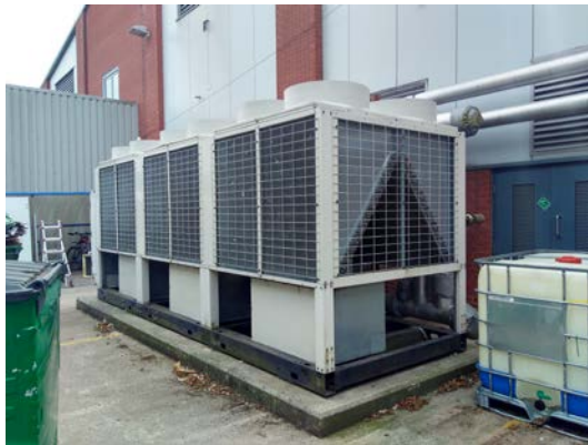
Figure 4 V-chiller near existing building
