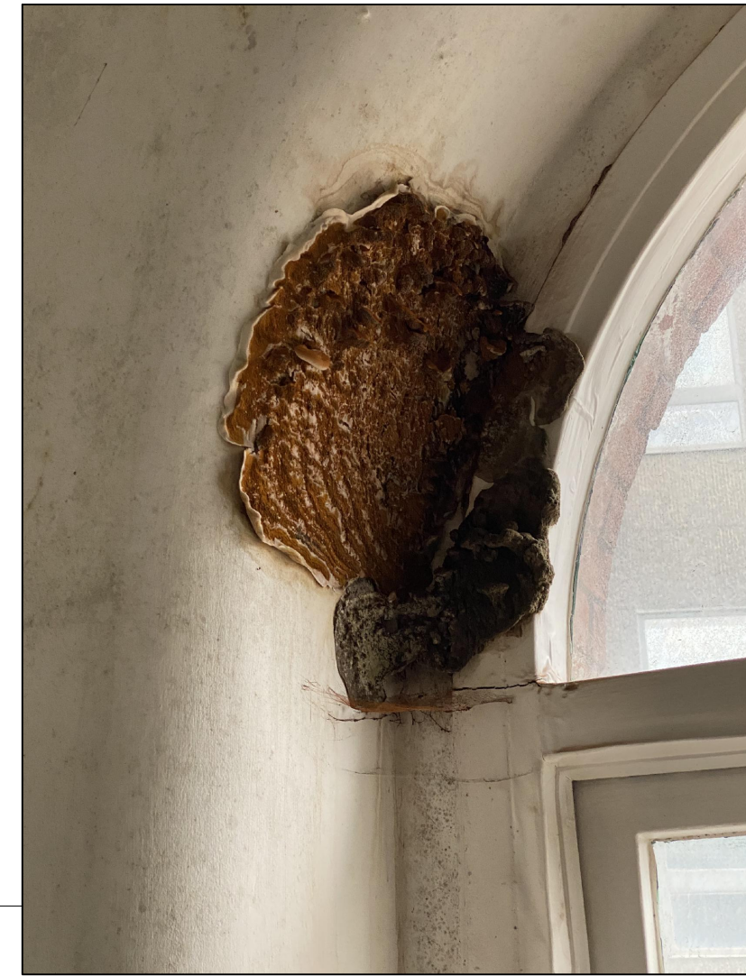
IMAGE 2 Any dry rot to be fully removed and repaired, walls replastered throughout
