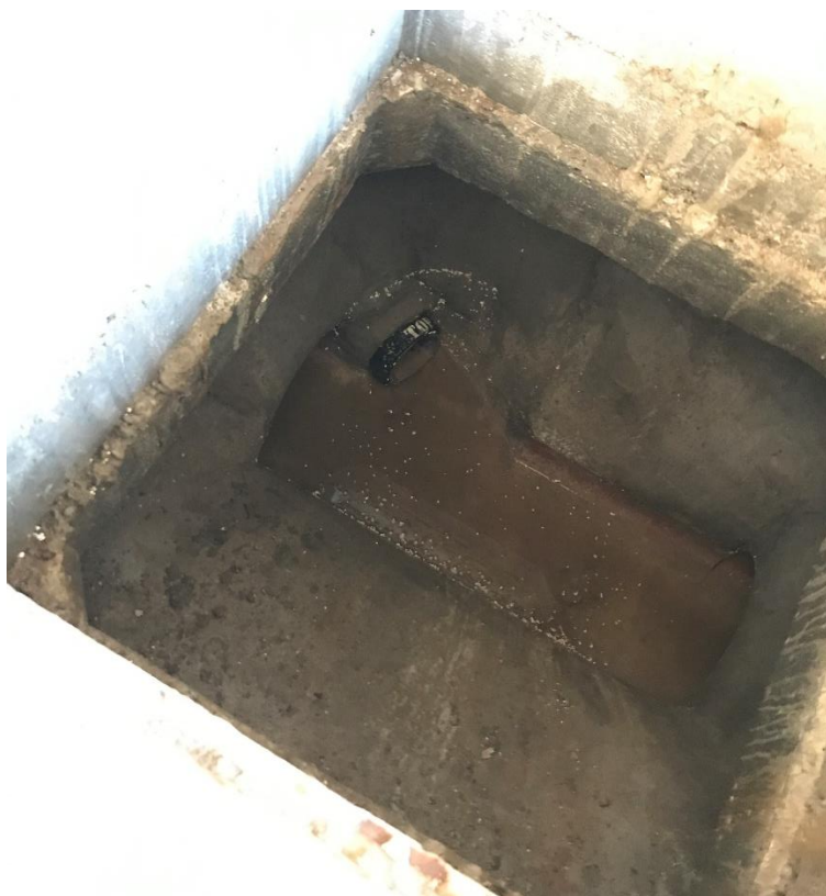
Photo 1 – As built Chamber
