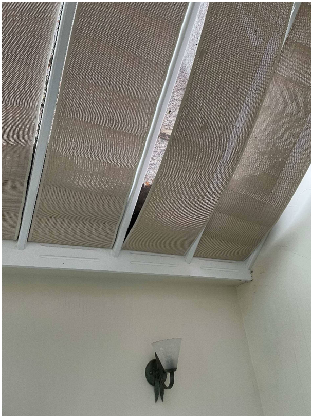
Photo 3. Internal photo showing build-up of leaves and debris in side gutter
