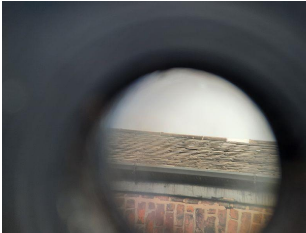
Plate 10: Lifted Tiles and Degraded Fascia to the South
