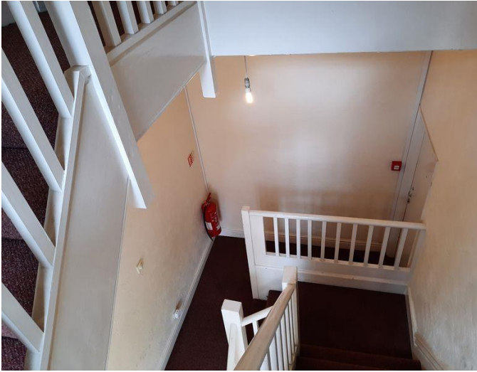
Plate 5: Narrow Corridors and Stairwells Leading to Flats
