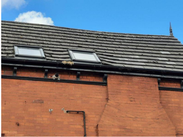
Plate 1: Dislodged and Warped Tiles Near Skylights
