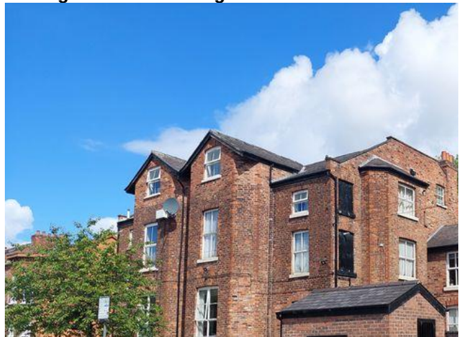
Plate 13: The South Of The Building with Worn Fascia Boards and Windows
