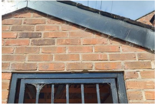
Plate 19: Cobwebbing along Fascia Boards
