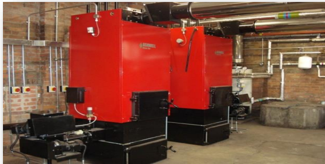
Plantroom Biomass Installation
