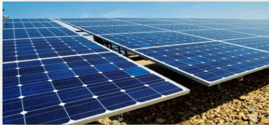
PV System components
