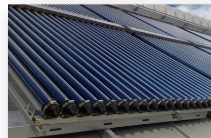
Example of Solar Thermal unit
