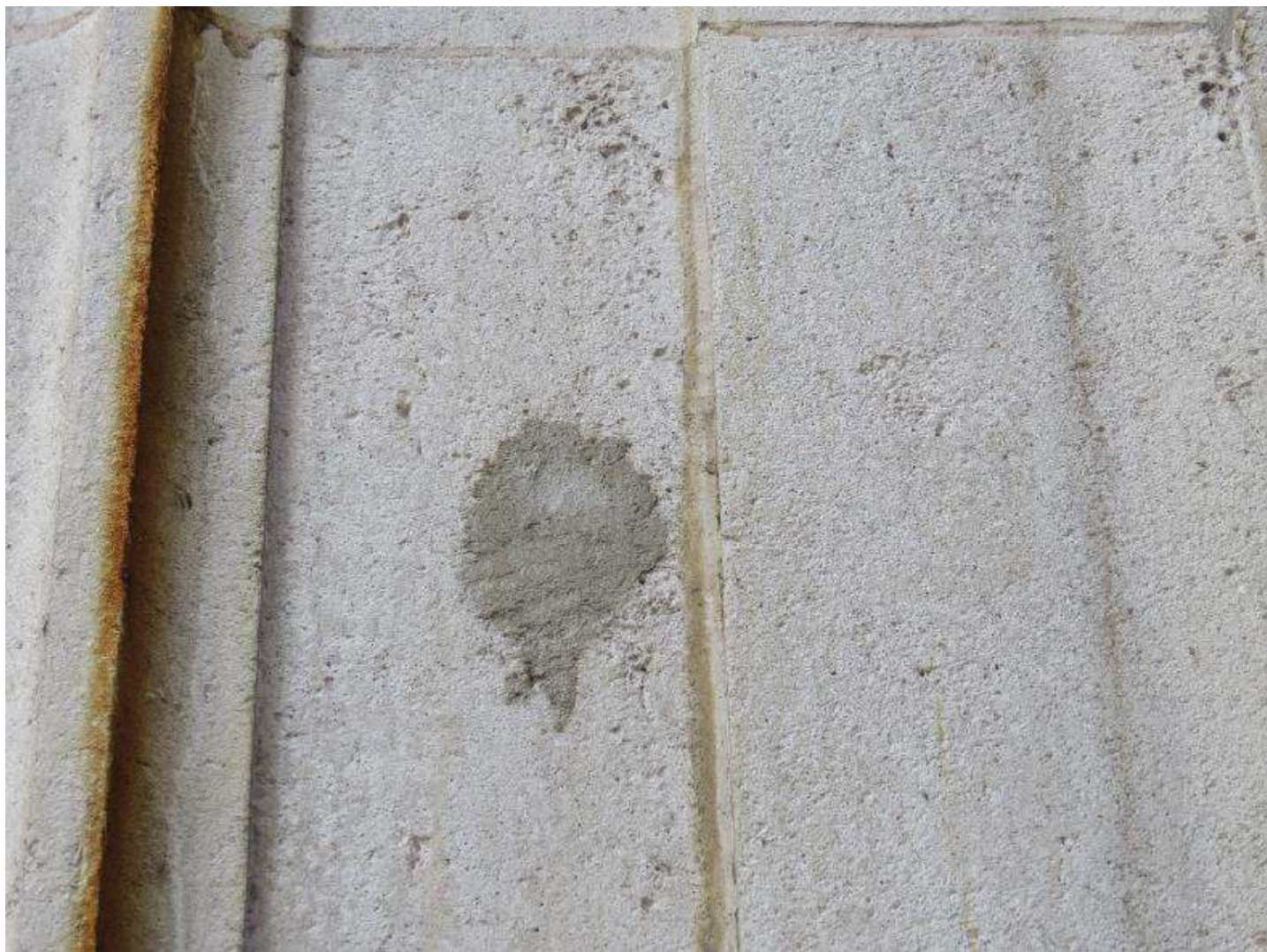
Fig. 9: The use of cement mortar repairs is inappropriate and where possible will need to be removed and replaced with a lime based mortar repair.
