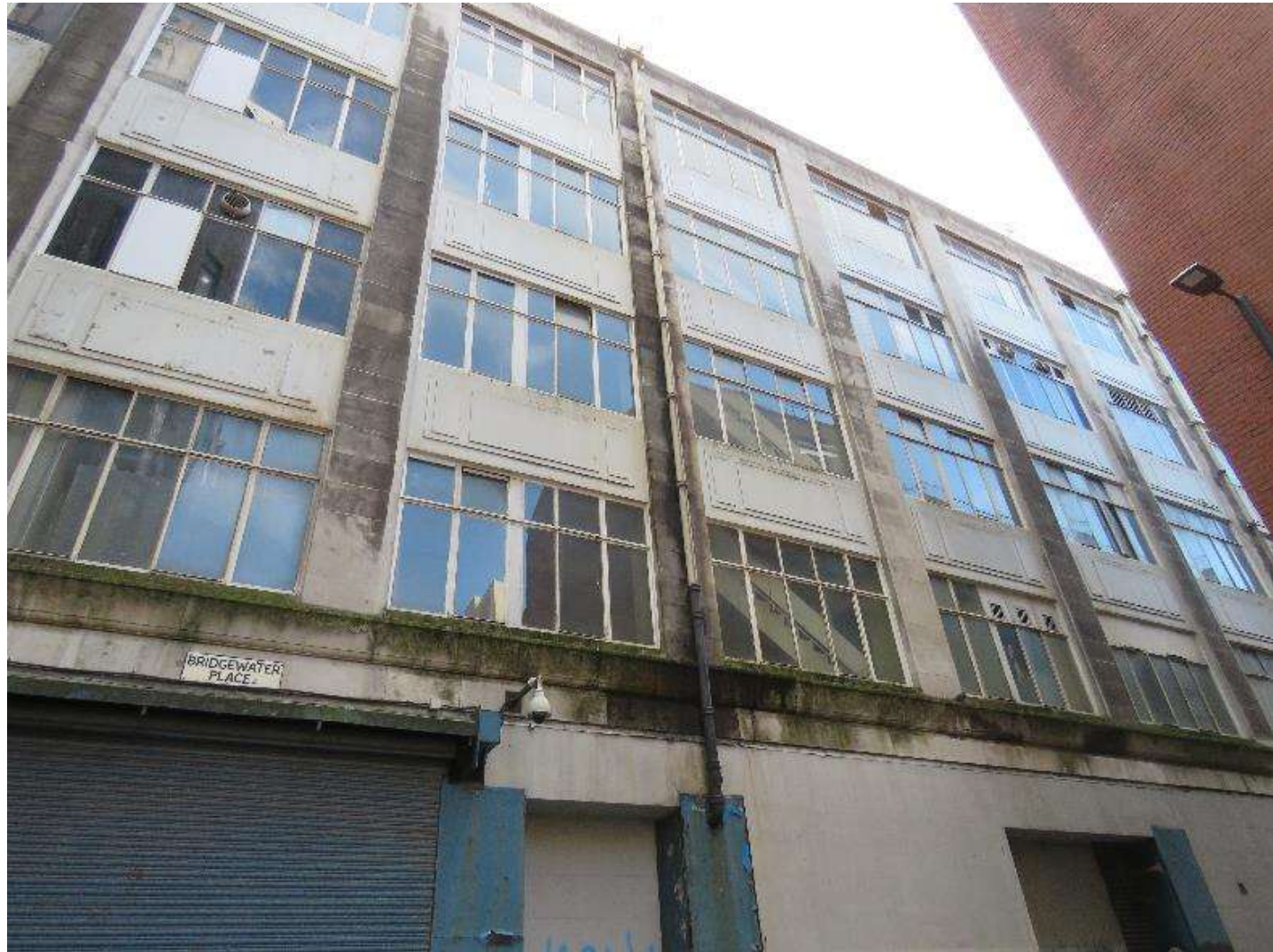
Fig. 7: View of the Portland limestone cladding to Bridgewater Place which has heavy soiling.
