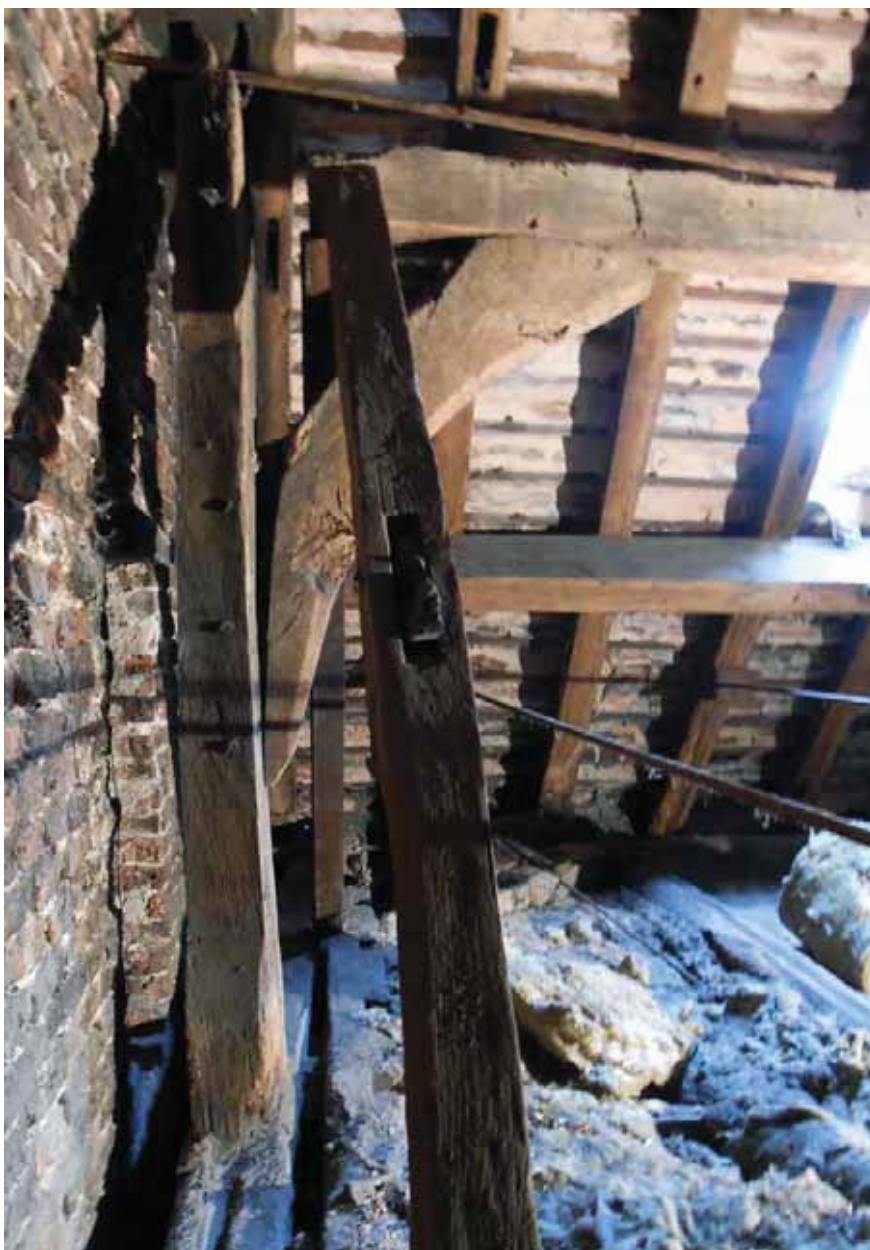
Plate 36. Bay 2, roof space, remains of northernmost crown post truss, viewed from west.
