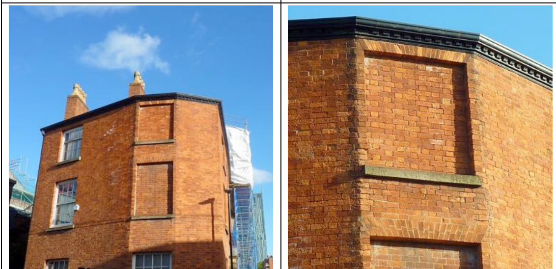
Upper wall is salt damaged and the mortar is washed out as the gutter overflows. Surplus water is penetrating the brickwork of the blank window infill.
