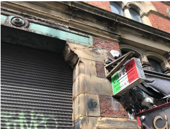
Spalled stone and masonry. (image taken prior to current works)
