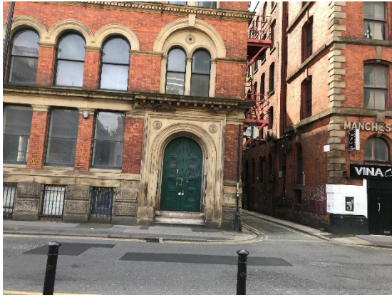
Front door to be overhauled and redecorated.
