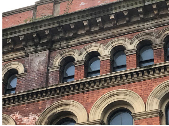
Water staining on the masonry at high level is to be investigated further.
