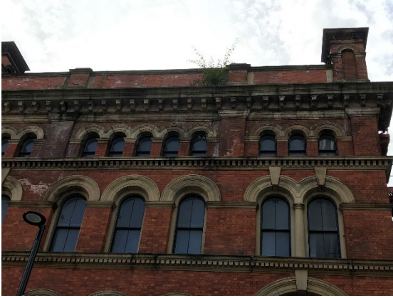
Vegetation to be removed and masonry repointed to cornice. See spec for outline description of new lead cladding to cornice.
