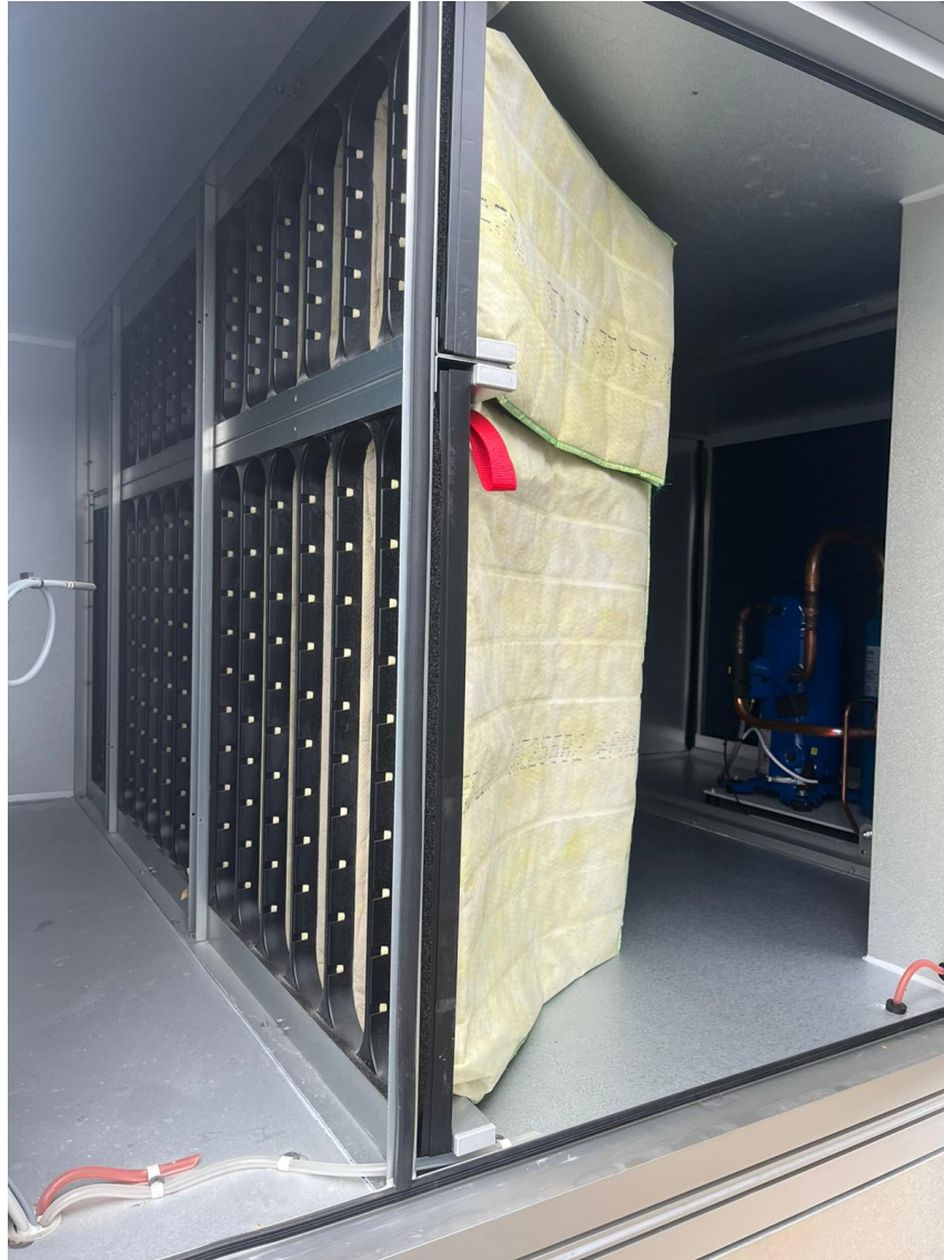
Figure 1-4 - Filter within AHU, accesable via access panel on the side of the unit at roof level
