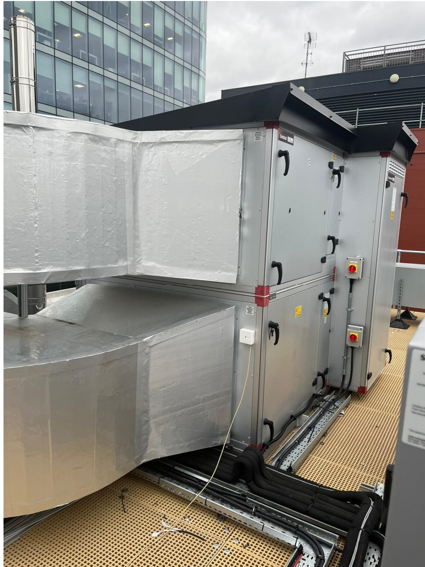
Figure 1-7 - Image of ductwork entering AHU
