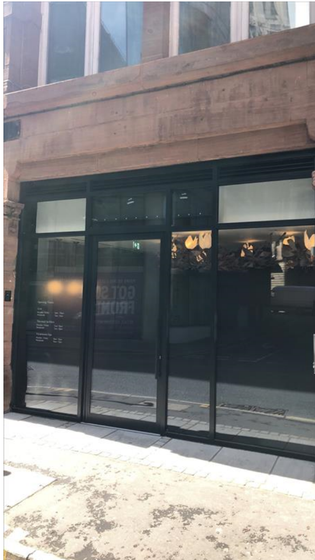
Figure 1-12 - Image of the kitchen extract louvre above the door
