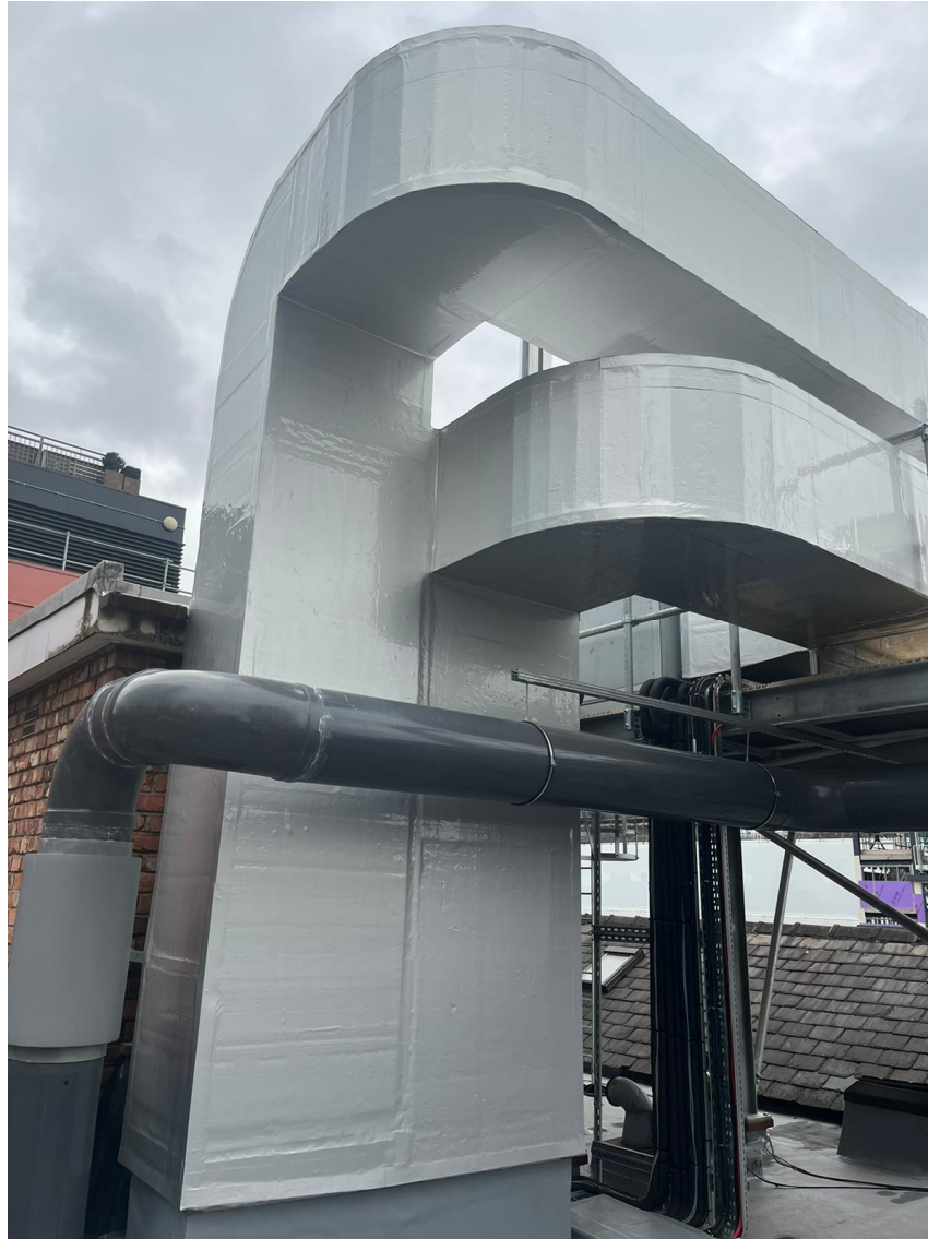
Figure 1-6 - Image of ductwork exiting the riser at roof
