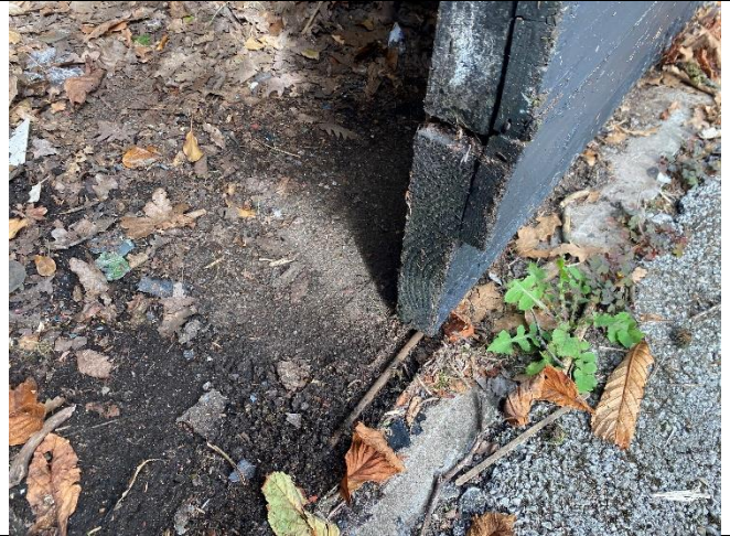
Existing door runner
