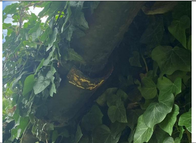
Displaced guttering requires repair
