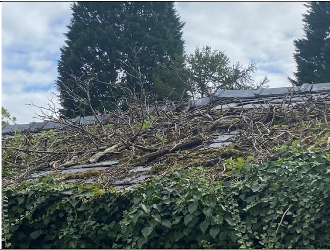
Roof repairs necessary to the rose garden elevation
