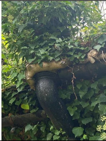
Rainwater goods blocked by Ivy
