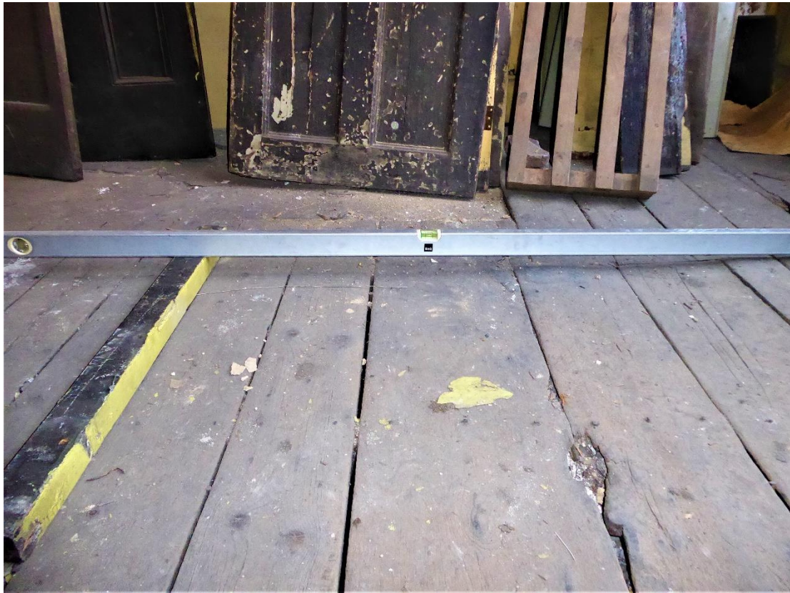
Photograph 11 – Showing the displacement of first floor at front of property.
