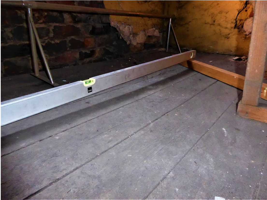
Photograph 8 – Showing displacement of second floor at the rear elevation
