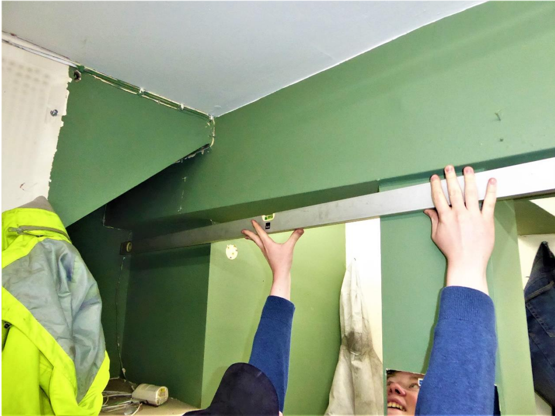
Photograph 16 – Showing deflection of supporting beam at ground floor ceiling level.
