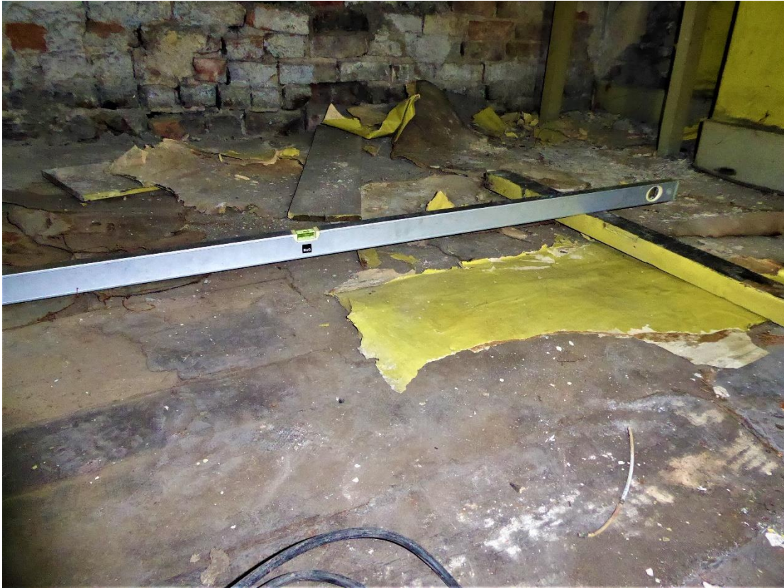
Photograph 14 – Showing displacement of first floor at rear elevation.
