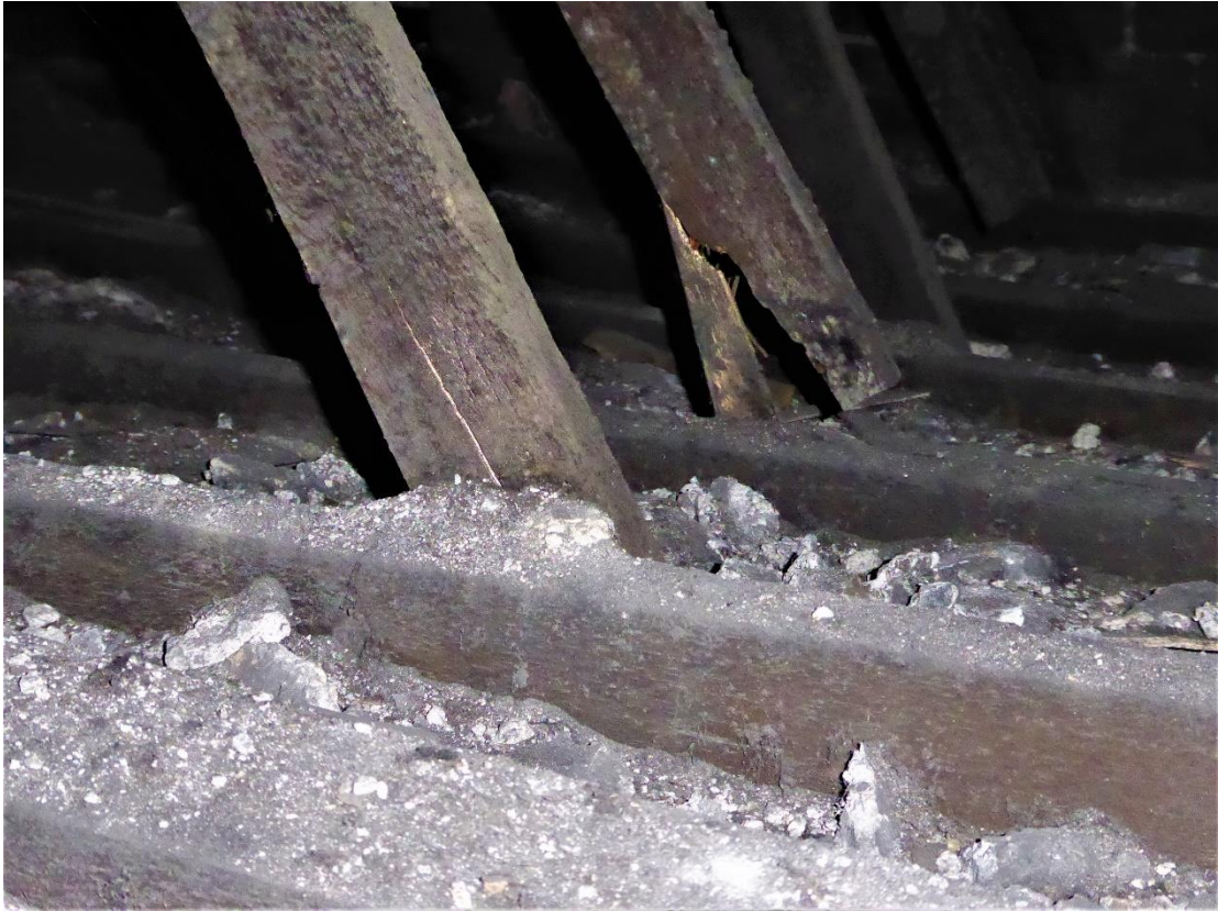
Photograph 4 – View of broken roof timbers.
