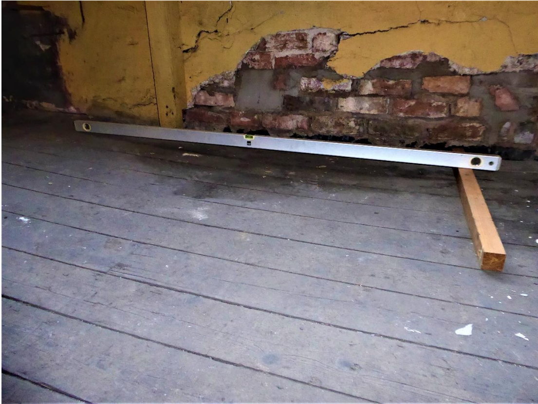
Photograph 9 – Showing displacement of second floor at the front elevation.
