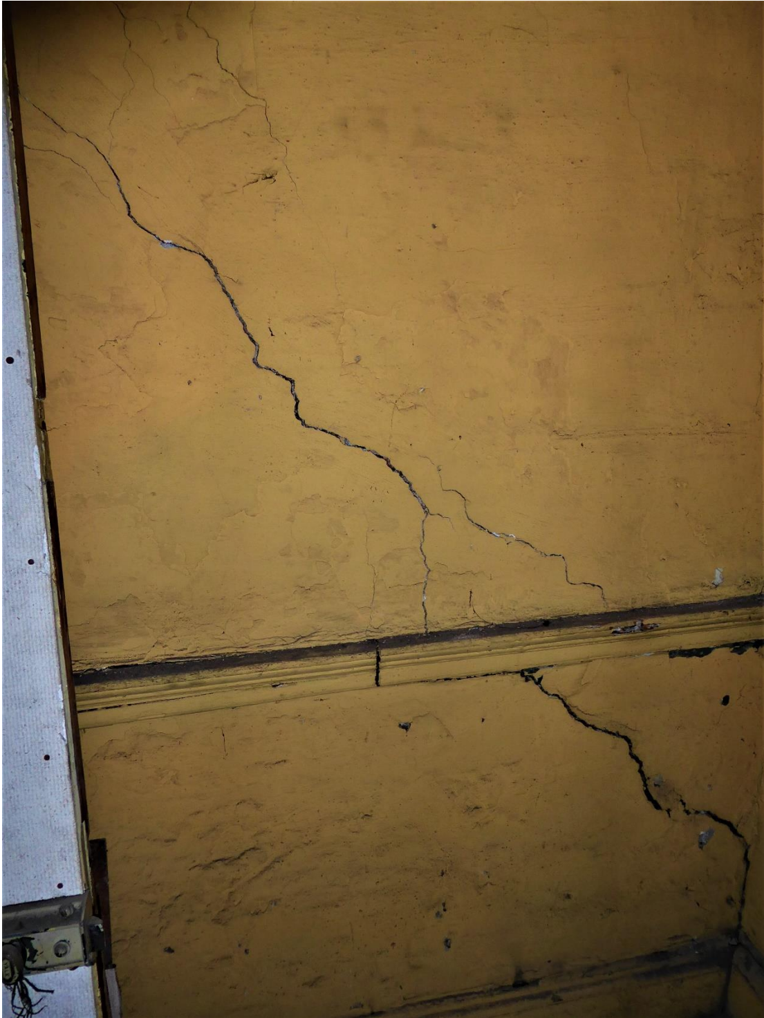
Photograph 12 – Showing movement cracks on internal wall at first floor level.
