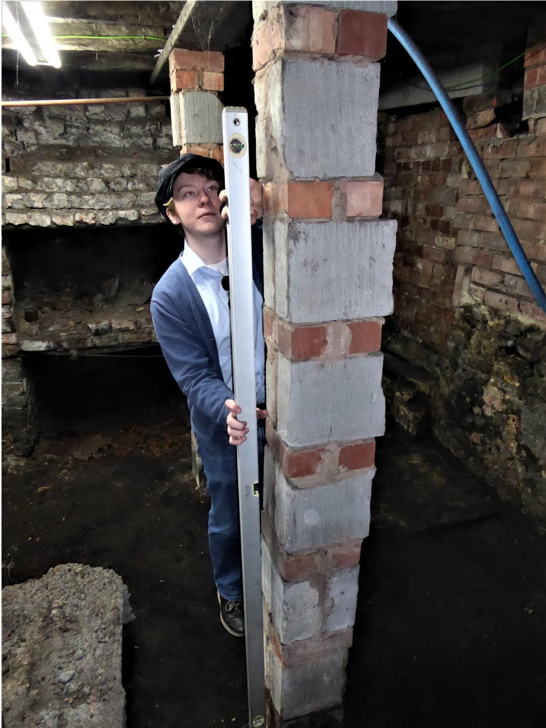
Photograph 19 – Showing poor construction of masonry piers in basement.
