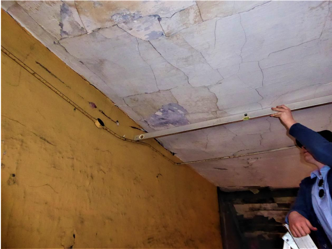
Photograph 5 – View showing sag in existing second floor ceiling.
