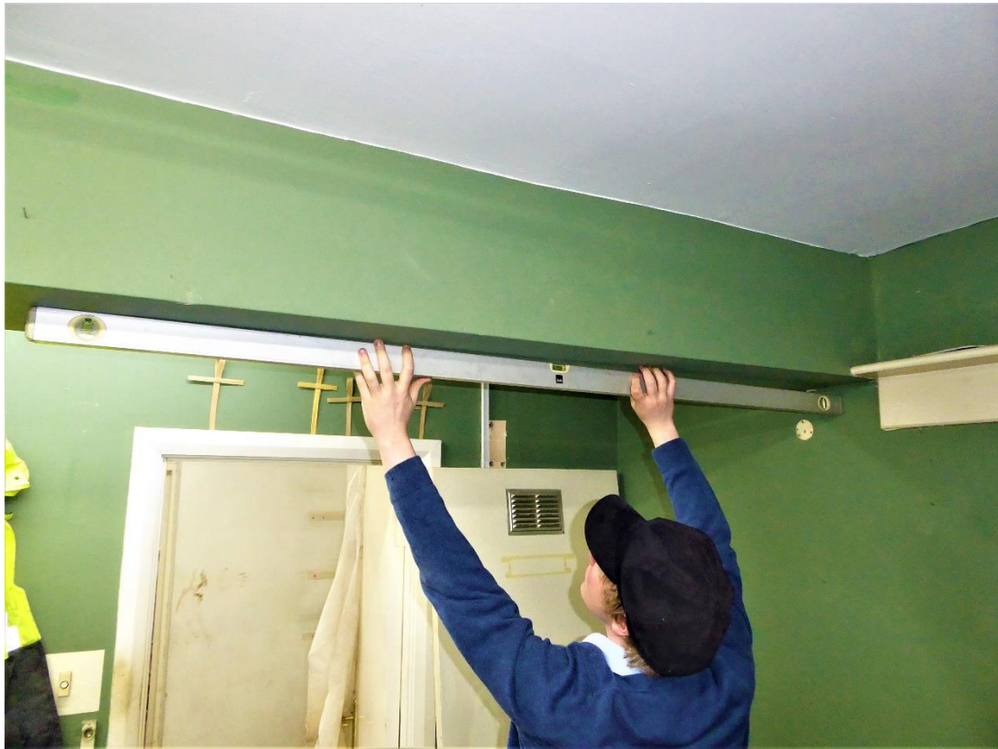
Photograph 15 – Showing deflection of supporting beam at ground floor ceiling level.
