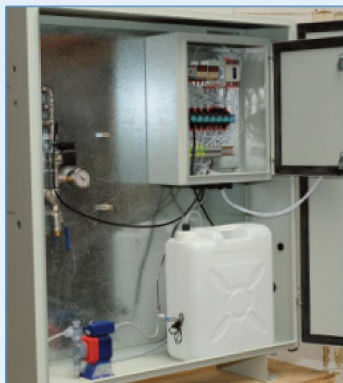
INTERIOR OF AUTOWASH CABINET
