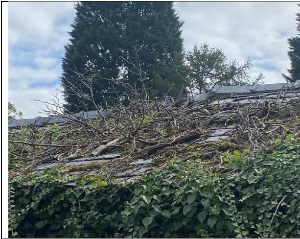
Roof repairs necessary to the rose garden elevation
