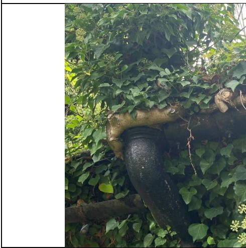
Rainwater goods blocked by Ivy
