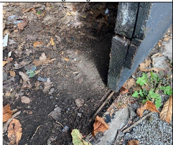
Existing door runner
