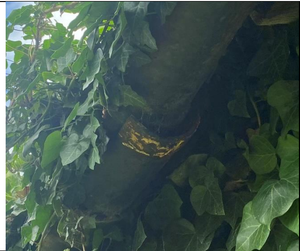
Displaced guttering requires repair
