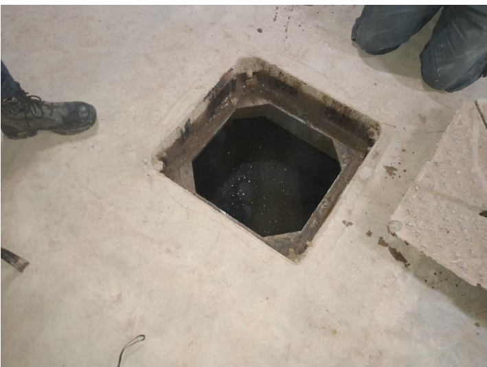
Photo 7 – SW09 Hydrobrake Chamber
