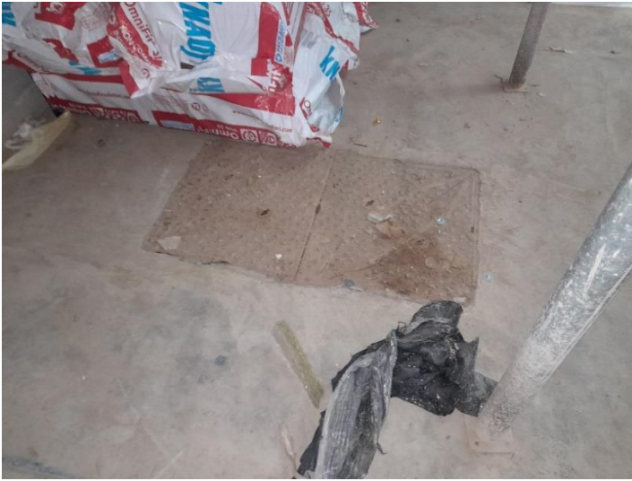
Photo 8 – FW07 – Type C Manhole Cover
