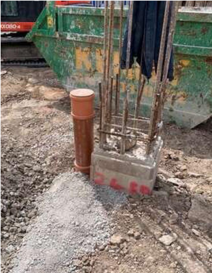
Photo 3 – Foul Pop-Up Adjacent Structural Columns
