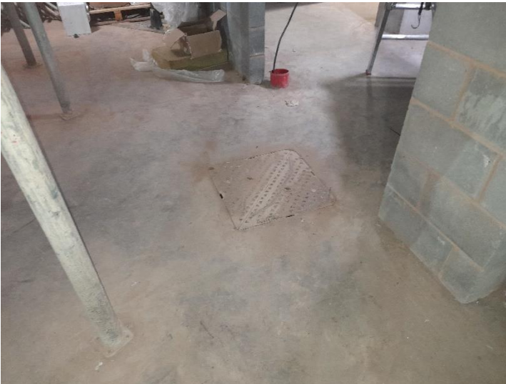
Photo 6 – FW08 Type B Manhole Cover
