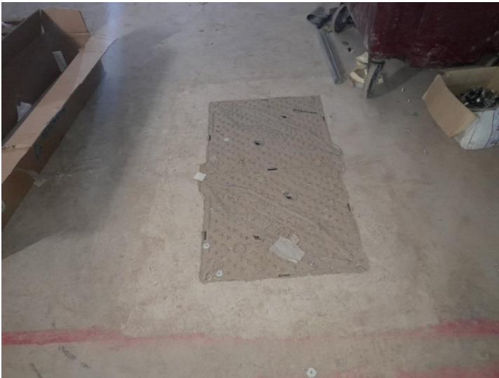
Photo 15 - FW04 Type C Manhole Cover
