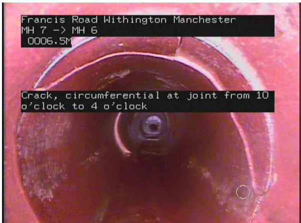
MH 7X_25292549-40df-401b-9bab-38cd316439f5_20210826_122 433_611.jpg, 00:00:58, 6.50 m Crack, circumferential at joint from 10 o'clock to 4 o'clock
