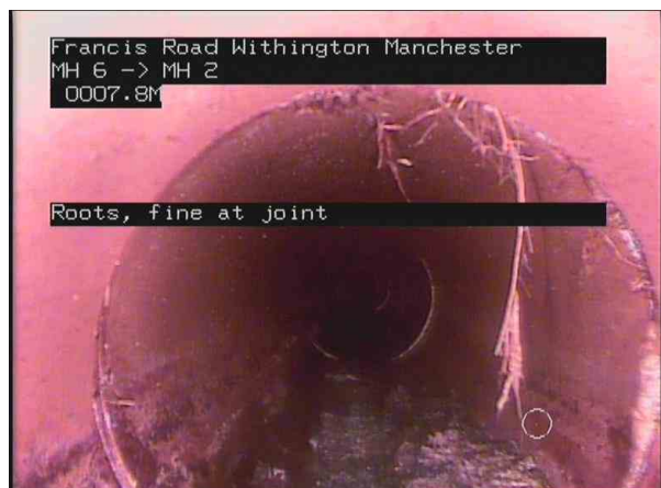
MH 6X_0c4209a3-33c5-41f5-bea8-fe52815a97e0_20210826_123 345_638.jpg, 00:01:44, 7.80 m Roots, fine at joint
