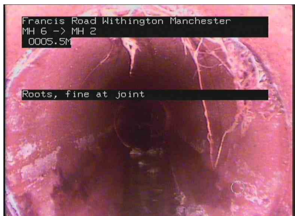
MH 6X_0931c0aa-7d6c-4dae-9774-04790d09fdf7_20210826_123 316_936.jpg, 00:01:24, 5.50 m Roots, fine at joint
