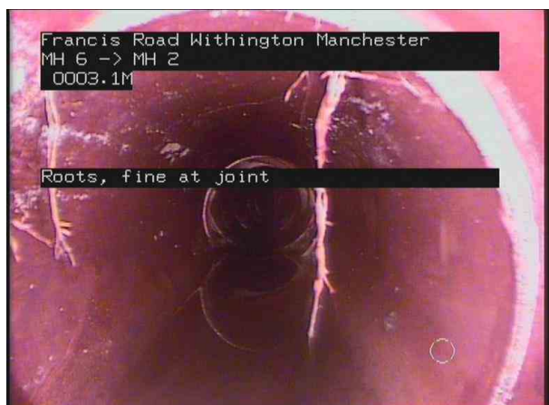
MH 6X_679ccf34-fa3f-4e8c-926d-a5e07571fd54_20210826_123234_241.jpg, 00:00:52, 3.10 m Roots, fine at joint
