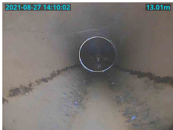
Branch AX_355f8f57-bb75-4385-89c4-08d93d51f94c_20210901_150 109_250.jpg, 00:00:41, 13.01 m Cracks, spiral from 8 o'clock to 1 o'clock
