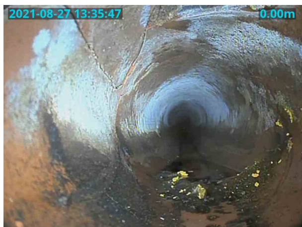
Branch AX_25e6c52b-56fe-439b-b680-e8e6e77cfe4a_20210901_154 701_639.jpg, 00:00:03, 0.00 m Crack, circumferential from 9 o'clock to 2 o'clock
