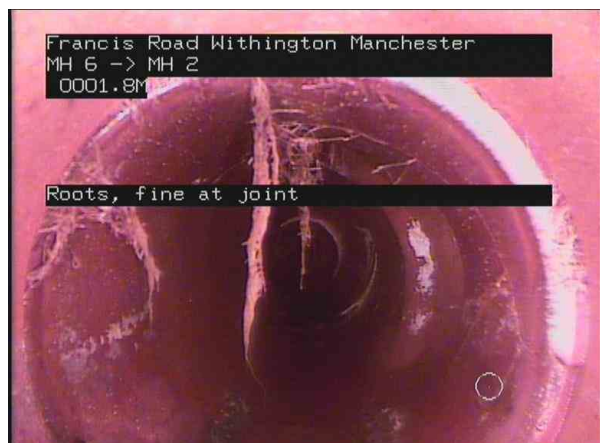
MH 6X_d6fb424a-92dd-4075-b6e5-791b967800ee_20210826_123208_276.jpg, 00:00:34, 1.80 m Roots, fine at joint
