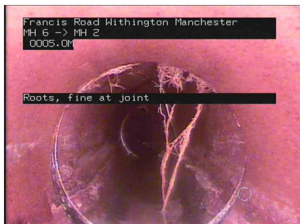
MH 6X_2b885c12-c565-4404-ab17-ac78dacc094_20210826_123305_219.jpg, 00:01:15, 5.00 m Roots, fine at joint
