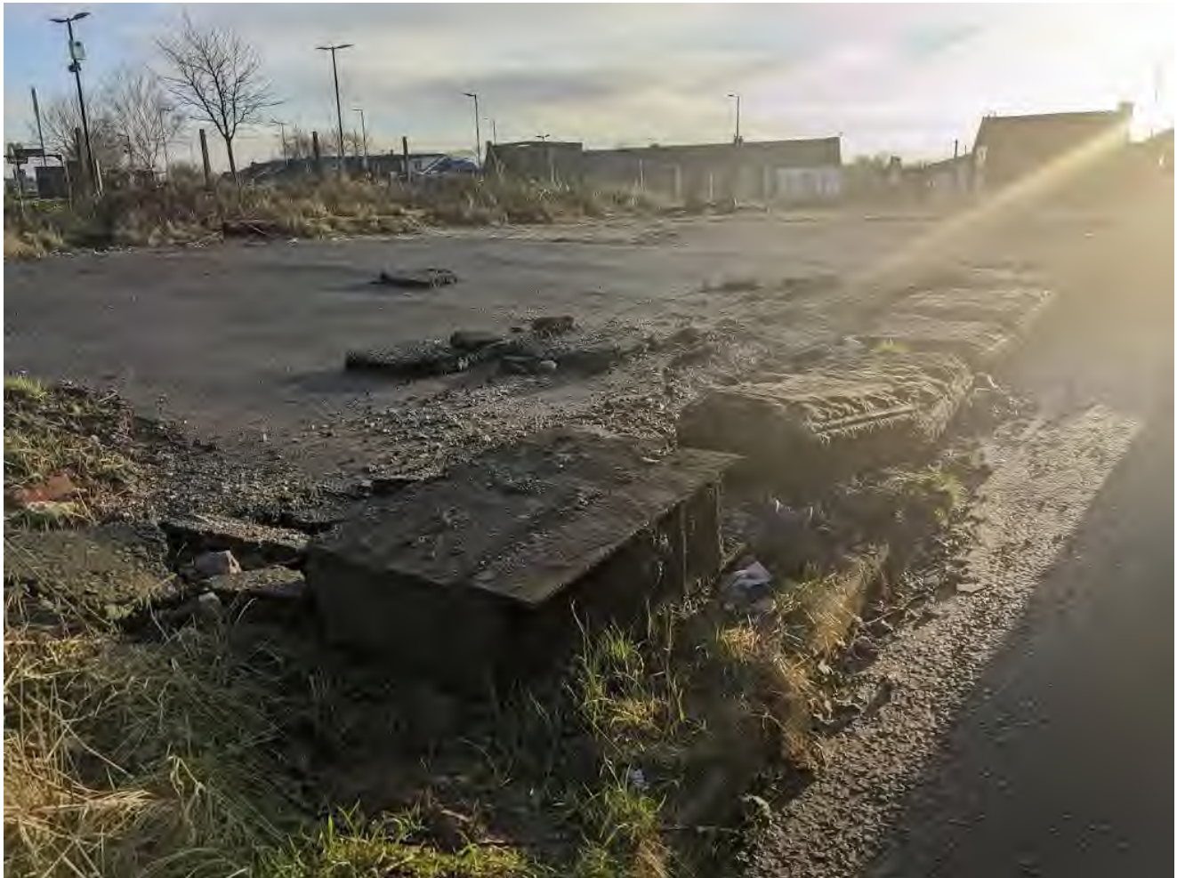
C2 – Demolition materials preventing vehicular access (looking southeast)
