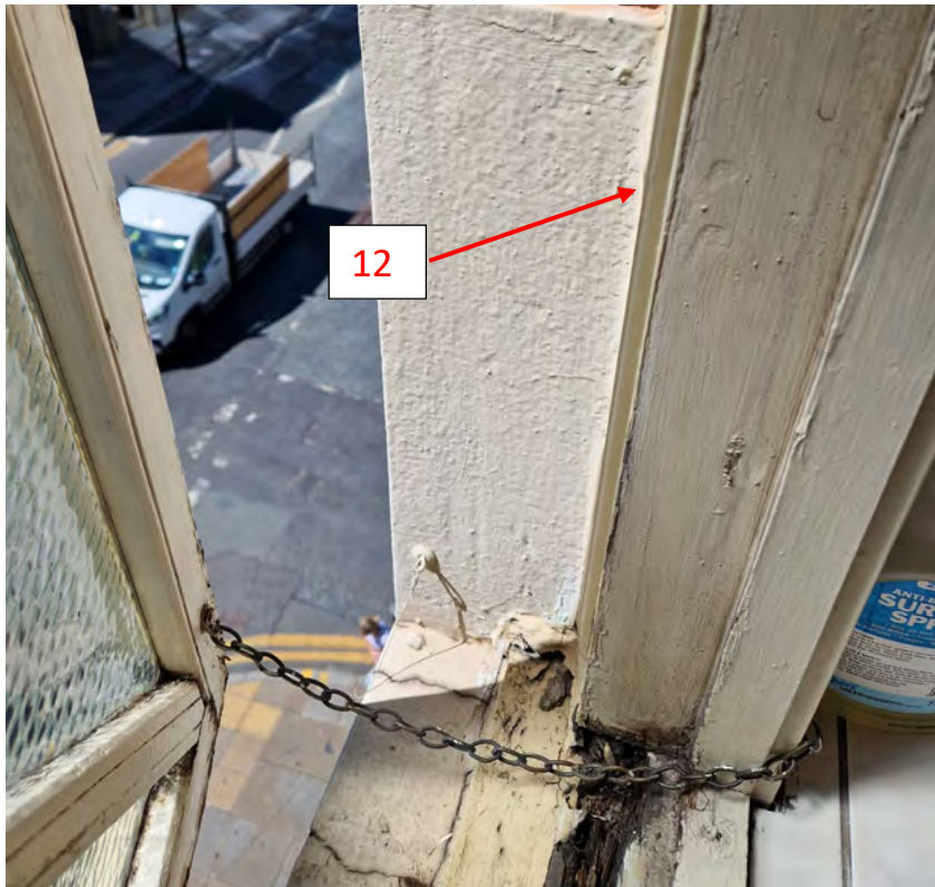
Figure 10: sample location 12 (upper window W8-LG)
