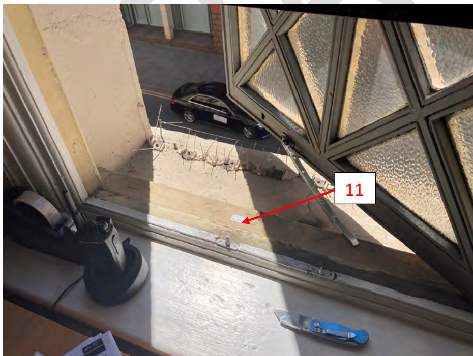
Figure 9: sample location 11 (upper window W11-LG)
