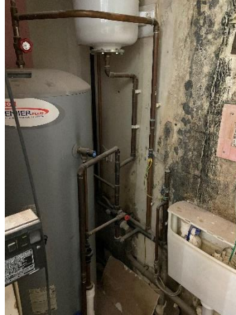
Photograph 32, Third Floor, Typical plant room
