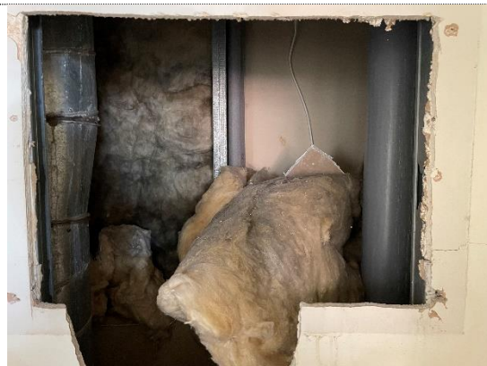
Photograph 24, First Floor, Typical SVP & ventilation duct boxed in
