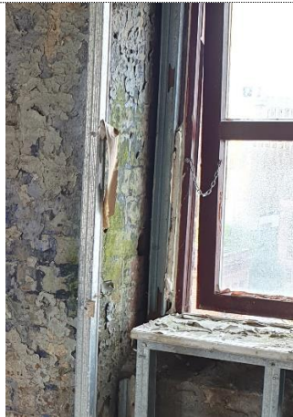
Photograph 40, Fourth Floor, Typical growing mold to external wall
