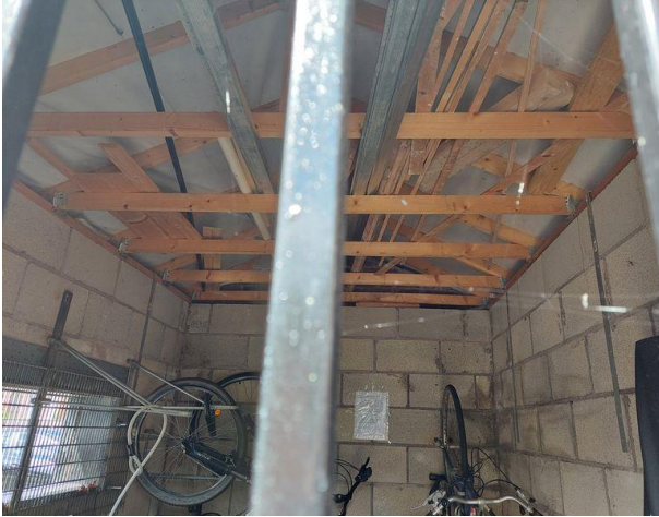
Plate 9.7: Breeze Block Inside with Wooden Supports
