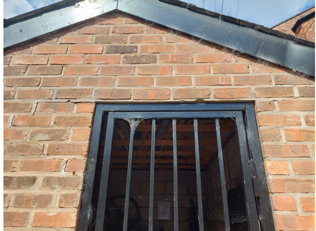
Plate 9.8 Wooden Fascia Boards on Bike Shed With Metal Grated Door, Open To Inside
