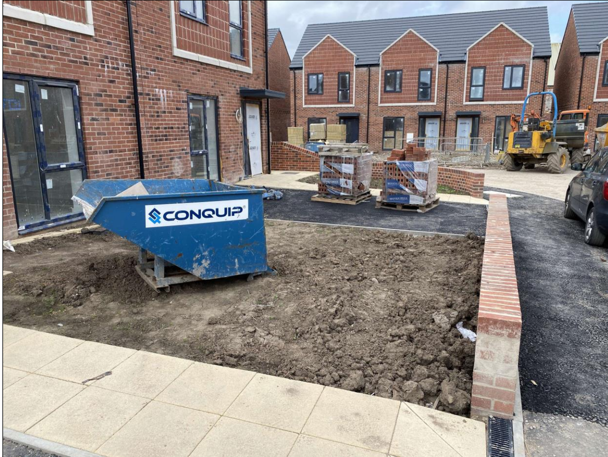
Photograph 10: Finished front garden area of plot 43.
