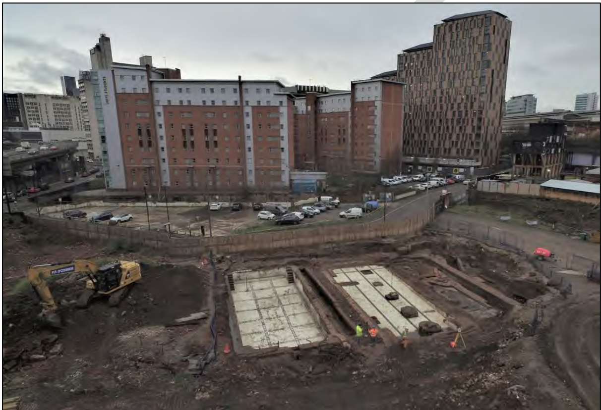
Plate xx: Aerial view of Mayfield Baths looking north-east
