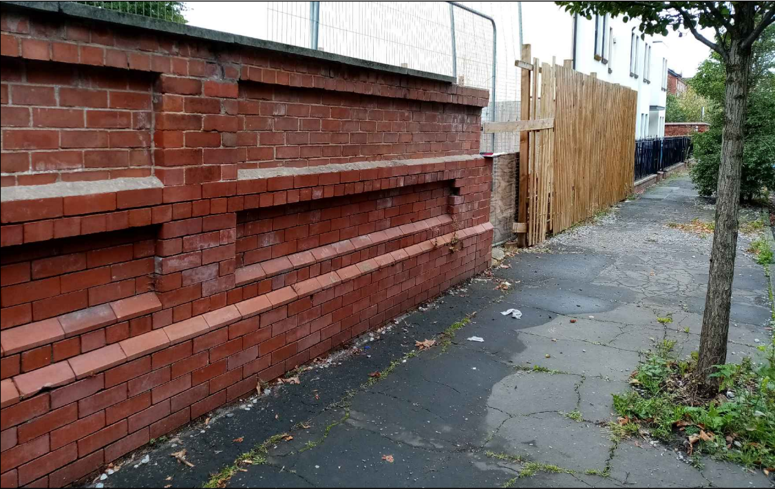
Proposed New Access Kerb Position - Showing current kerb in dilapidated state
