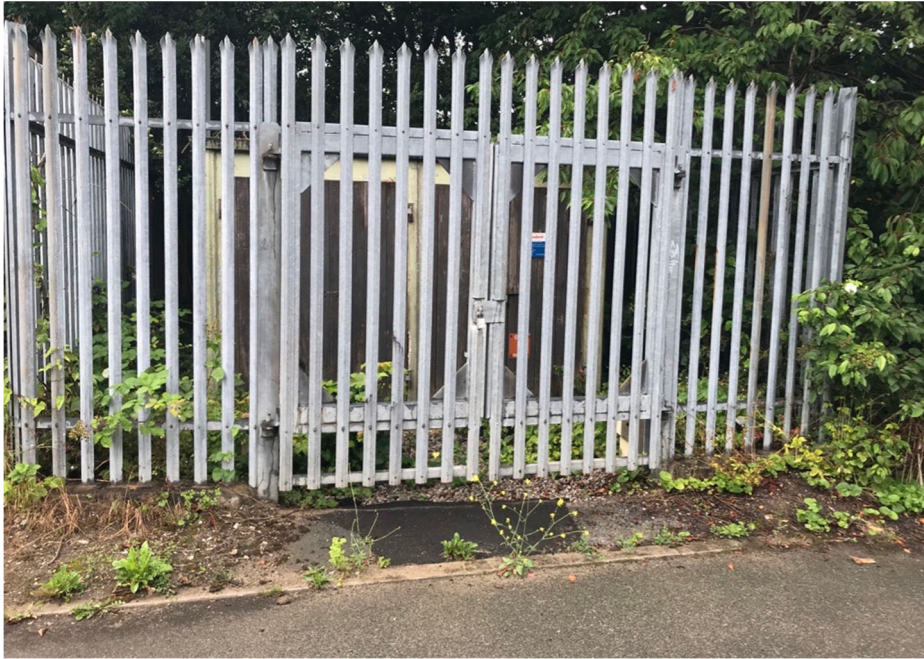
Figure 2: The existing gas governor site (Google Earth Streetview, 2021)
