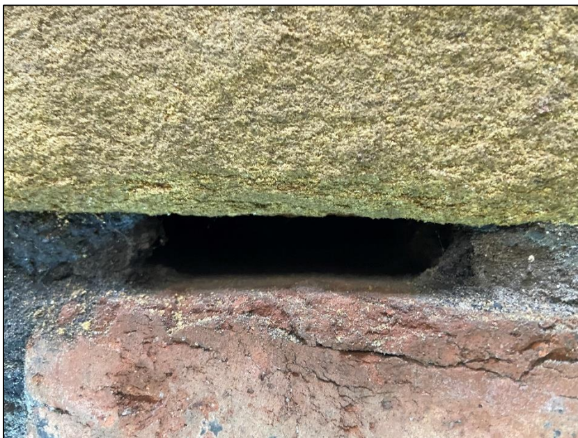
Photograph 15 showing the shallow cavity within the brickwork
