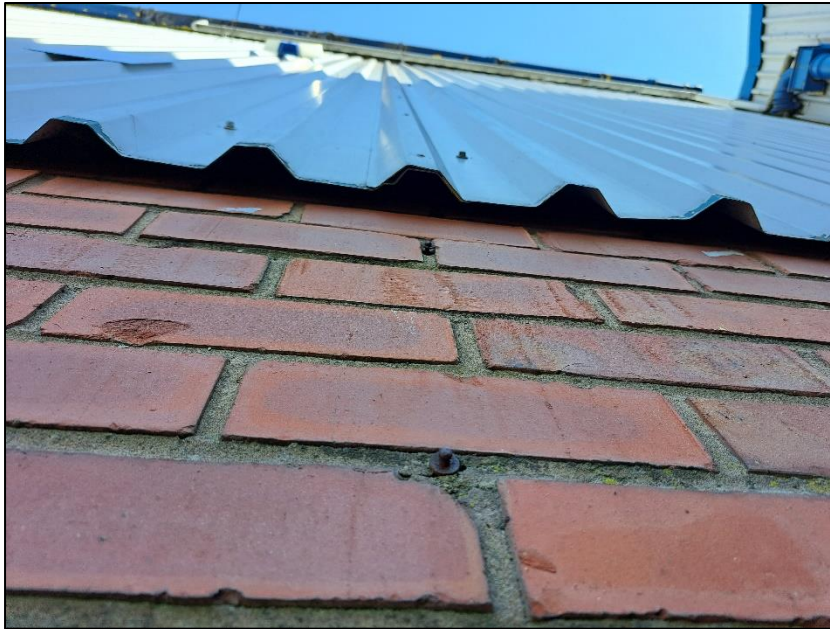
Photograph 6 showing the gap between the brickwork and the metal cladding
