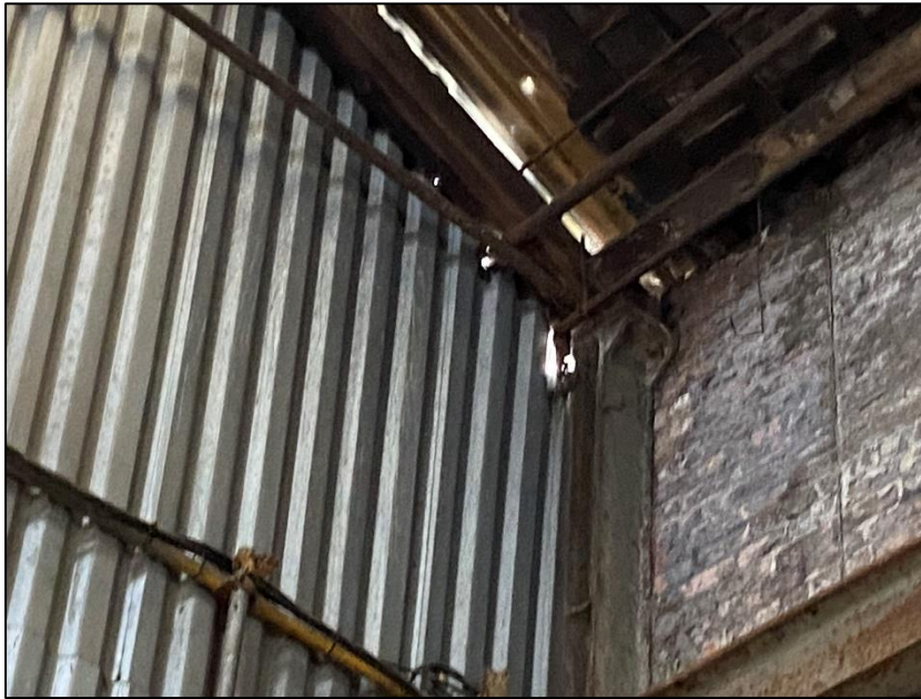
Photograph 16 showing the daylight at the roof edge
