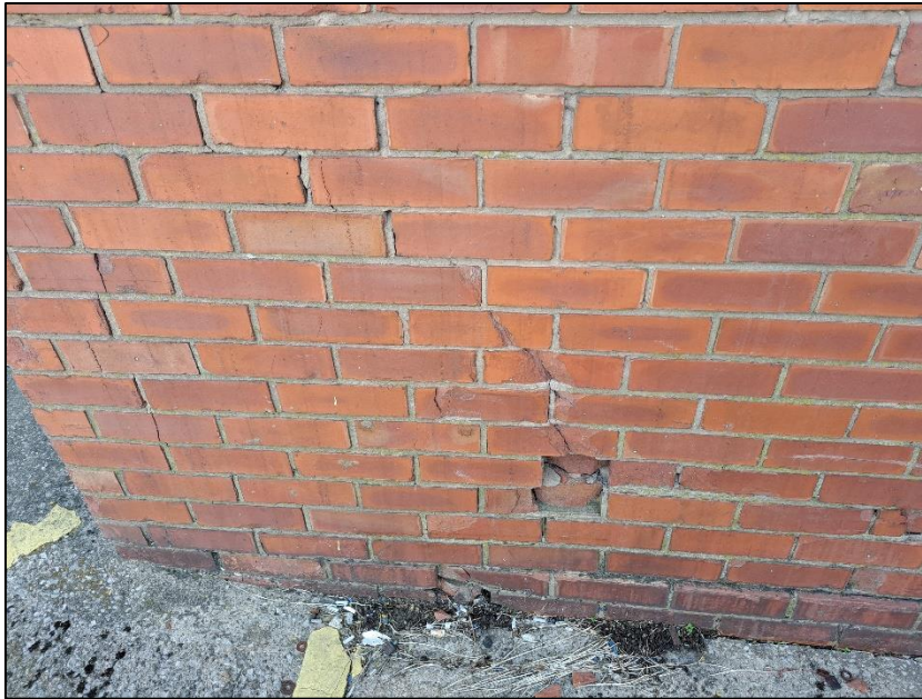
Photograph 4 showing an area of superficial damage on the brick section of the walls
