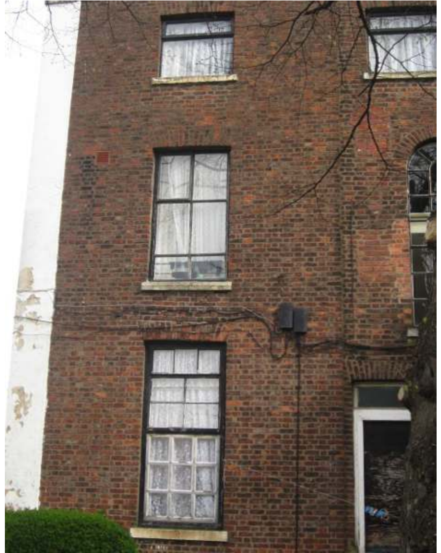
inappropriate windows to rear elevation
