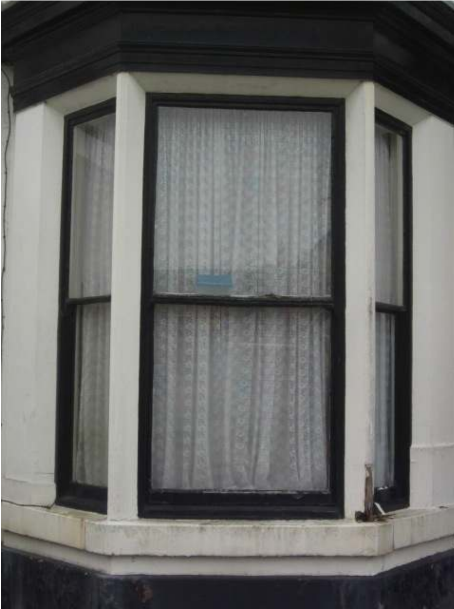
Timber Bay window with Sash window showing signs of rot.
