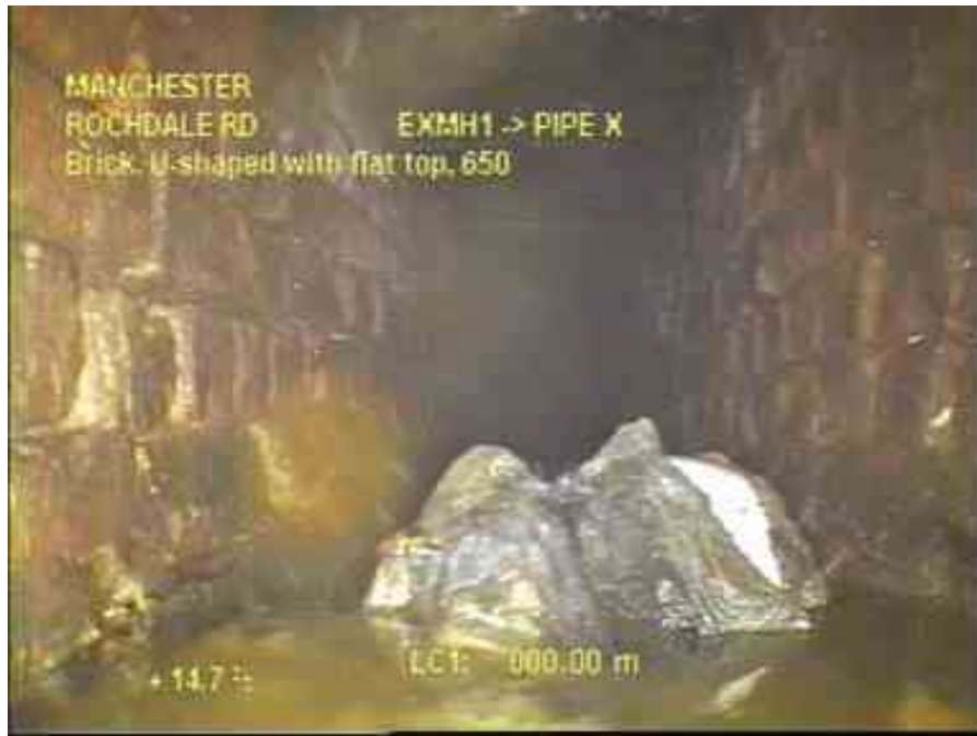
1, 00:00:19, 0.60 m Settled deposits, hard or compacted, 25% cross-sectional area loss, COMPACT DEBRIS / CONCRETE
