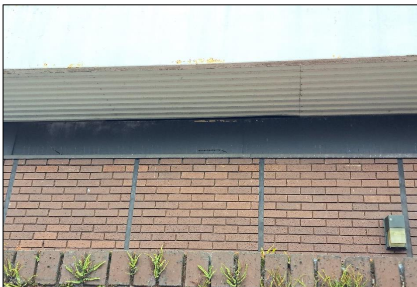
Photograph 12 showing a small gap between the capping and brickwork
