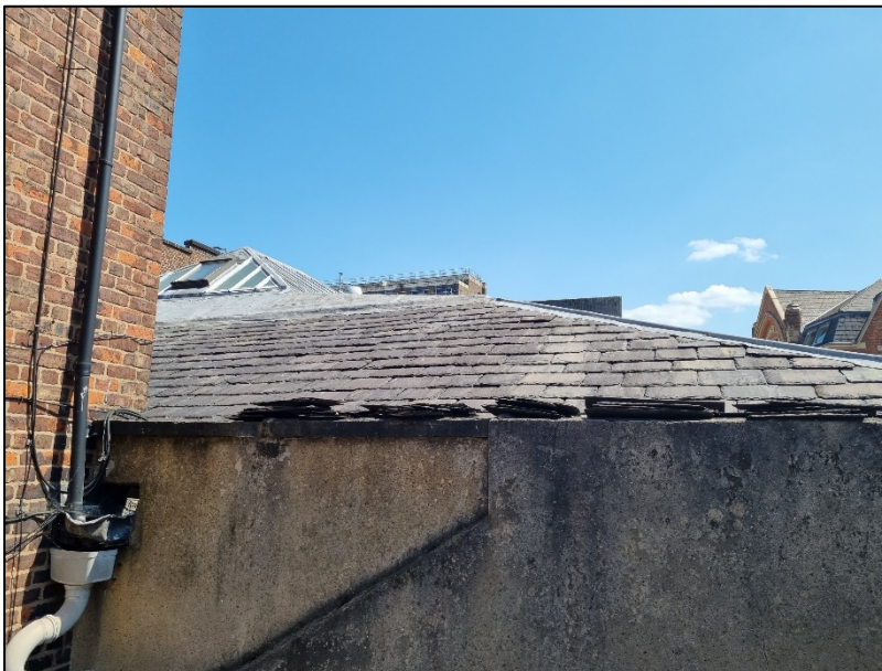
Photo 3 Slate roof tiles of B1 showing gaps
