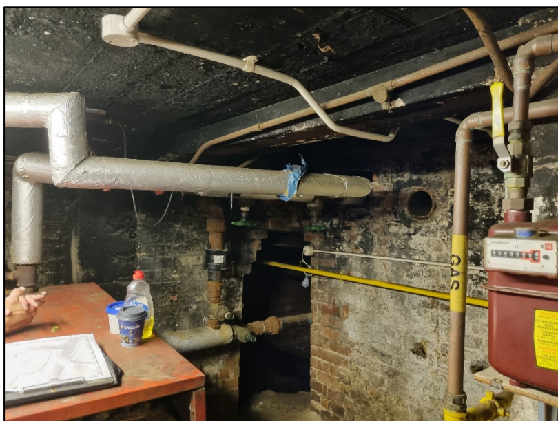
Photo 6 Dark cellar with gaps and crevices within the brick work
