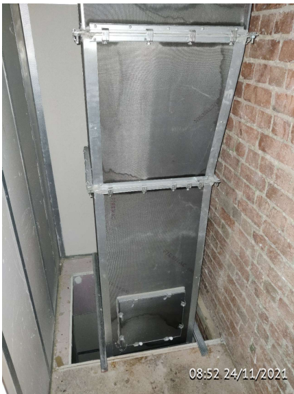
Kitchen Extract Riser - Supplied Rated Ducting To Roof
