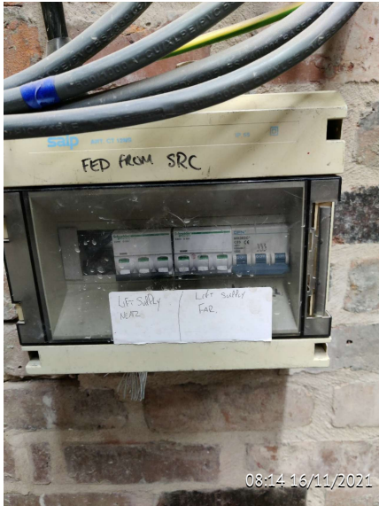
'Lift Supply' Board
