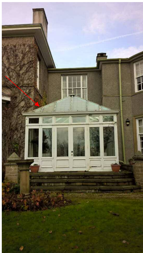
Photo 6. Highlighting side gutter which becomes heavily blocked with leaves and debris
