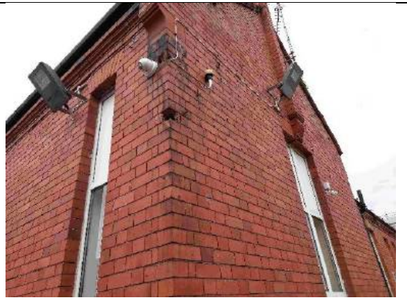
Photograph 16: Missing brickwork on B4
