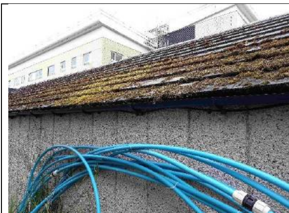
Photograph 5: Dense moss coverage on roof of garages (B1)
