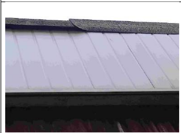
Photograph 13: Lifted felt on roof of B3
