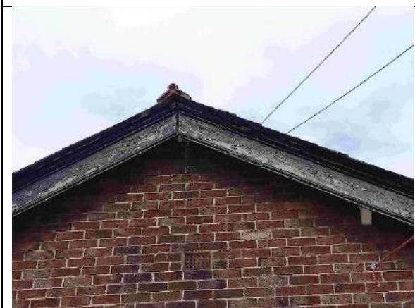
Photograph 19: Gap at gable end of B5a
