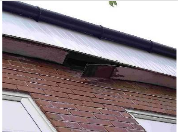
Photograph 12: Broken soffit board on B3
