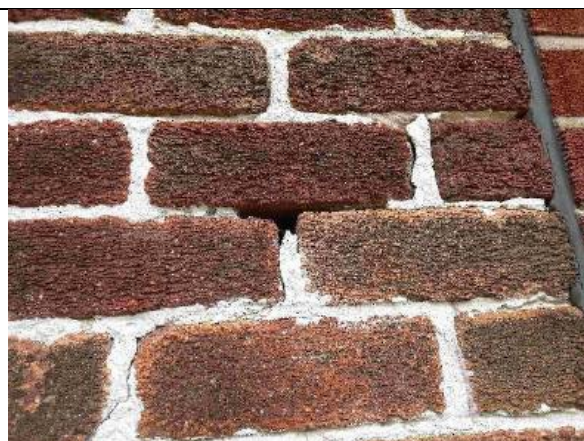
Photograph 7: Missing mortar on B2
