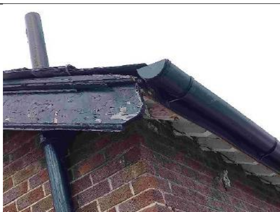
Photograph 18: Gaps between roof tiles and facias on B5a
