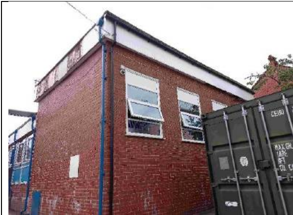
Photograph 11: Broken fascias on building B3
