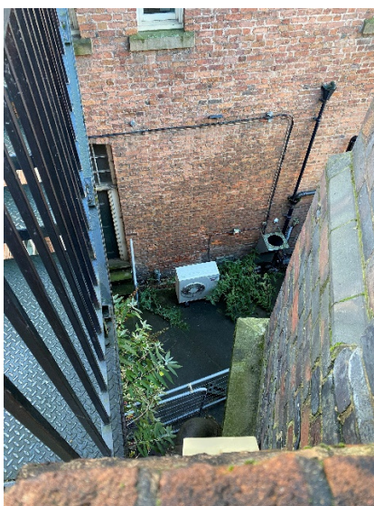
Image 5: Existing heat pump location
