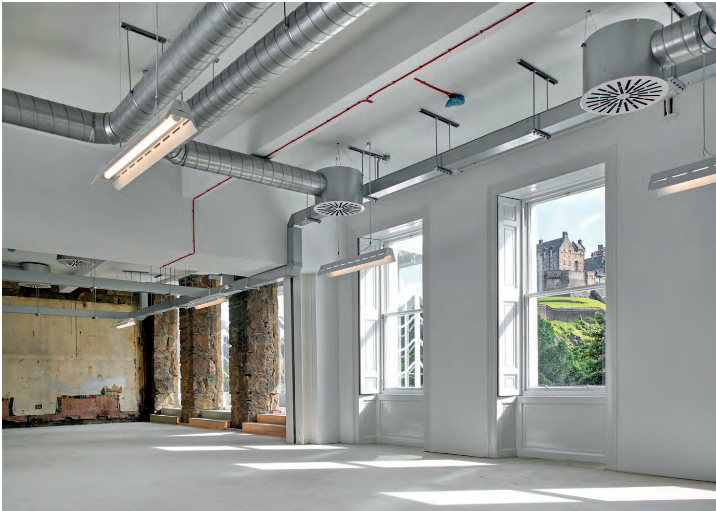
White soffite with aluminium ductwork
