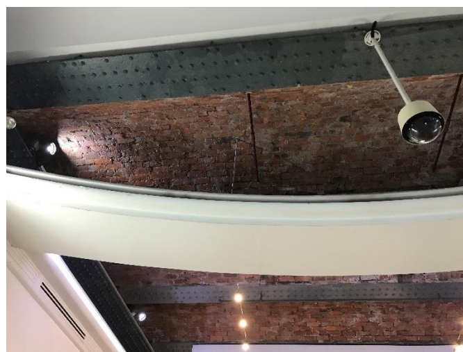
Figure 6.4: Existing tie rods installed at Level 01
