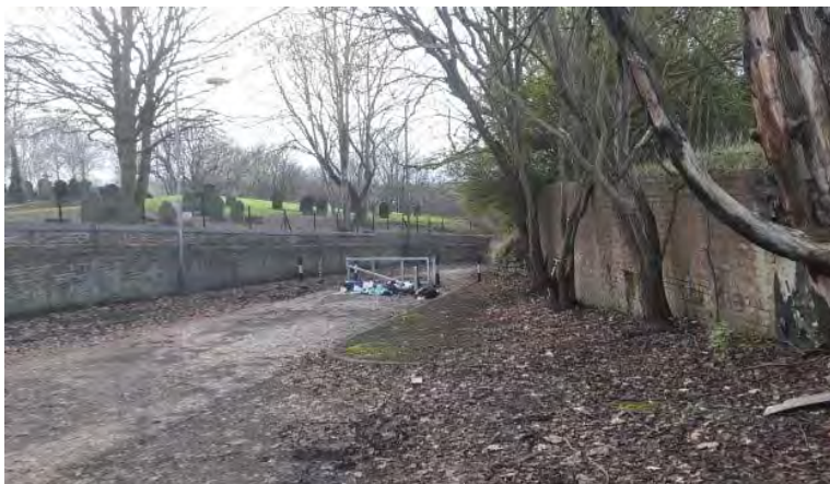
Photograph 6 (P6) Retaining wall and off-site fly tipping to the south of the site.
