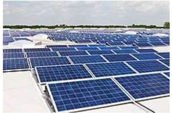
Figure 8 Example of Rooftop Solar PV
