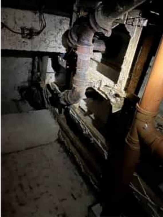
Photo 5, Drainage located in basement - RE2
