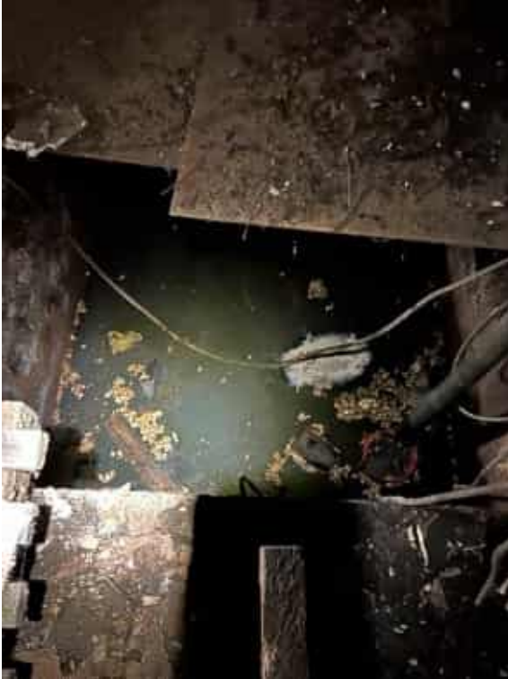
Photo 12, Sump pit located in basement - pumps out to MH2. Believed to be abandoned and disconnected.
