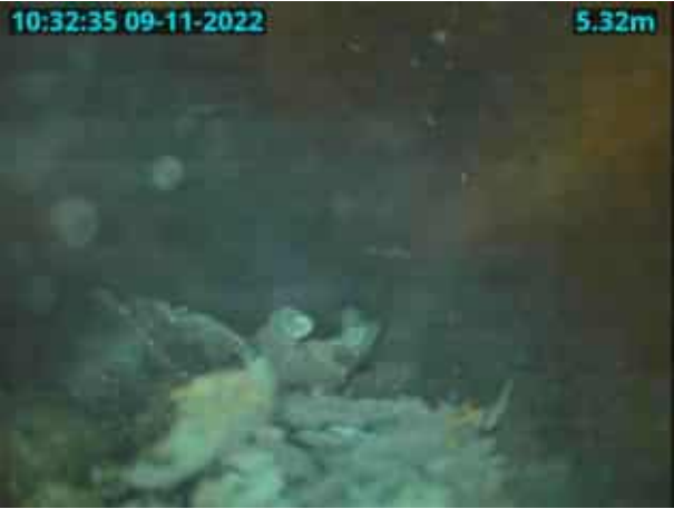
RE 1X_529feaf0-5f7e-4972-b3bc-b78d09d2556a_20221126_103453_712.jpg, 00:00:38, 5.32 m Settled deposits, fine, 10% cross-sectional area loss
