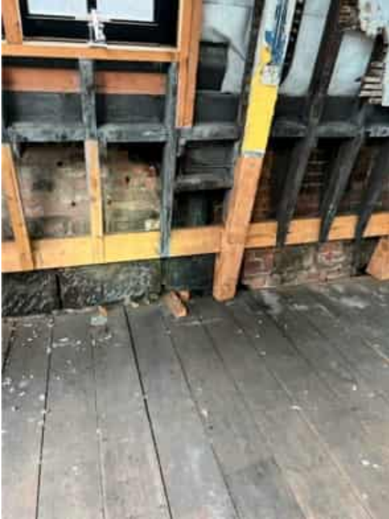
Photo 10, Rainwater pipe hoppers located on the top floor of the building, all discharge directly down to below ground drainage. No access points to rainwater pipes.
