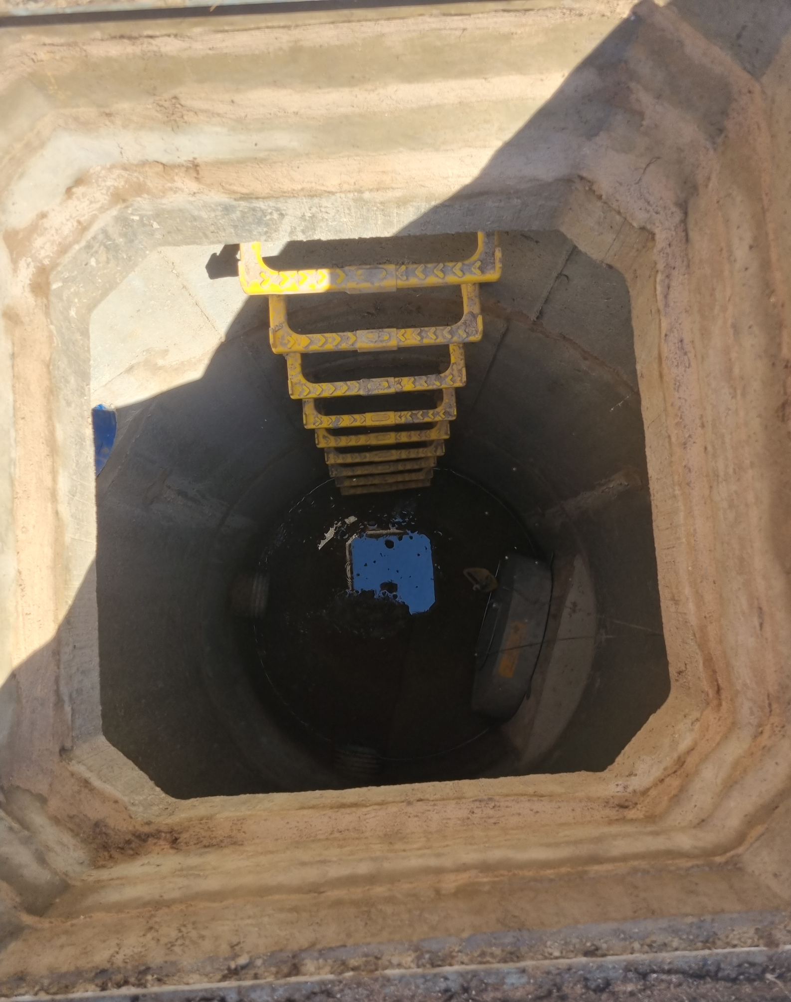
FLOW CONTROL INSTALLED IN SWMH046
